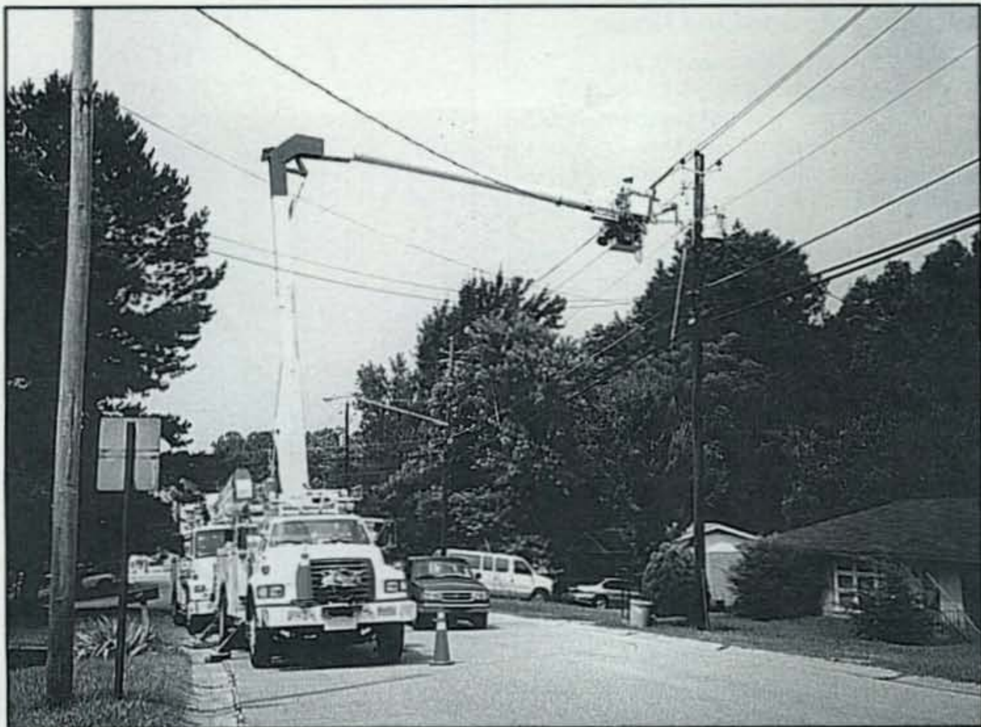
Photo D— The final results and ultimate reward! Here two crews from a local power company replace aluminum clamps and a lightning arrestor on a “noisy pole”— and eliminate an S9 noise level located with an MFJ-852 Line Noise Meter.
