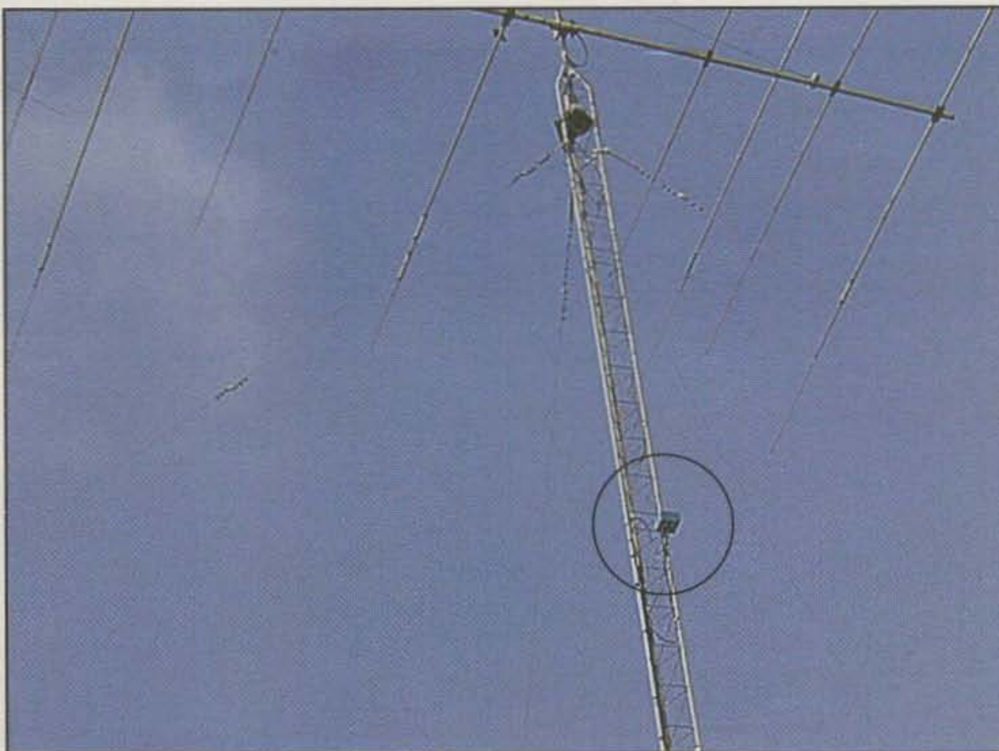
Photo C— The StackMatch outside box was mounted at 80 feet on a tower leg using the U-bolt provided.
