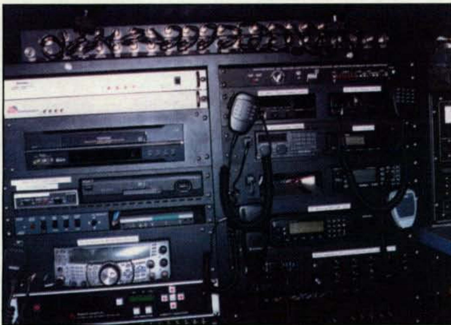
Interior view of the Red Cross communications response vehicle. Gear includes HF, VHF, and UHF transceivers usable as needed both on and off the ham bands. (WB6NOA photo)
