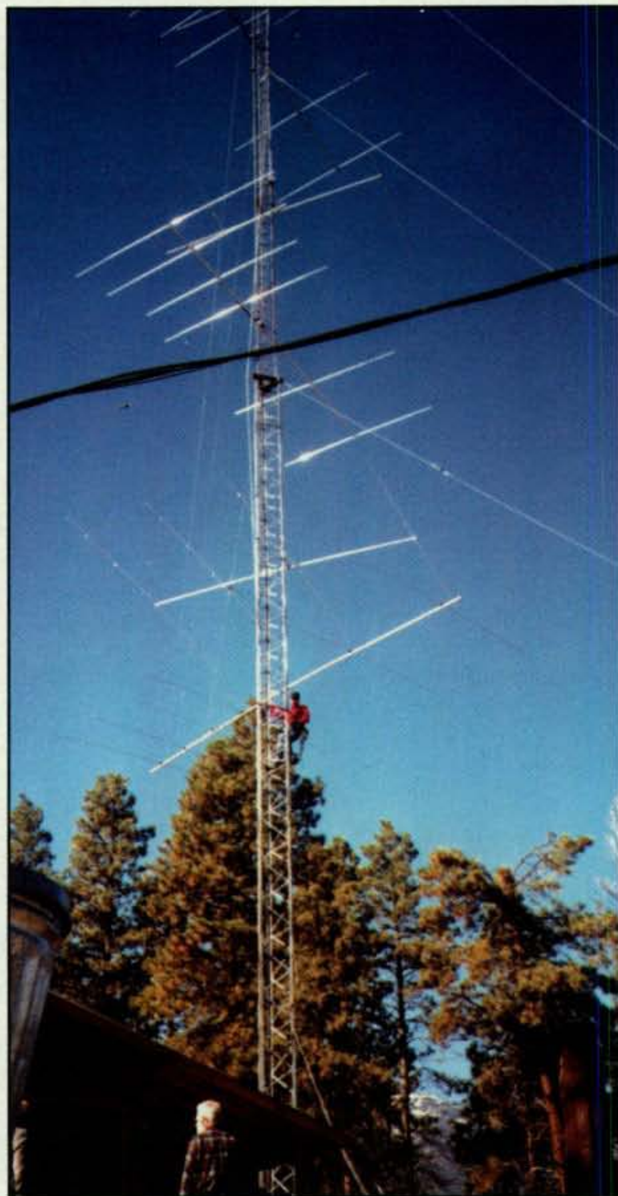
You don't have to have a super antenna system like this, but it helps. Very large and complex antenna systems are used at winning contest stations. Multiple transceivers connected to multiple tower and antenna systems are built to maximize signals in desired directions.
