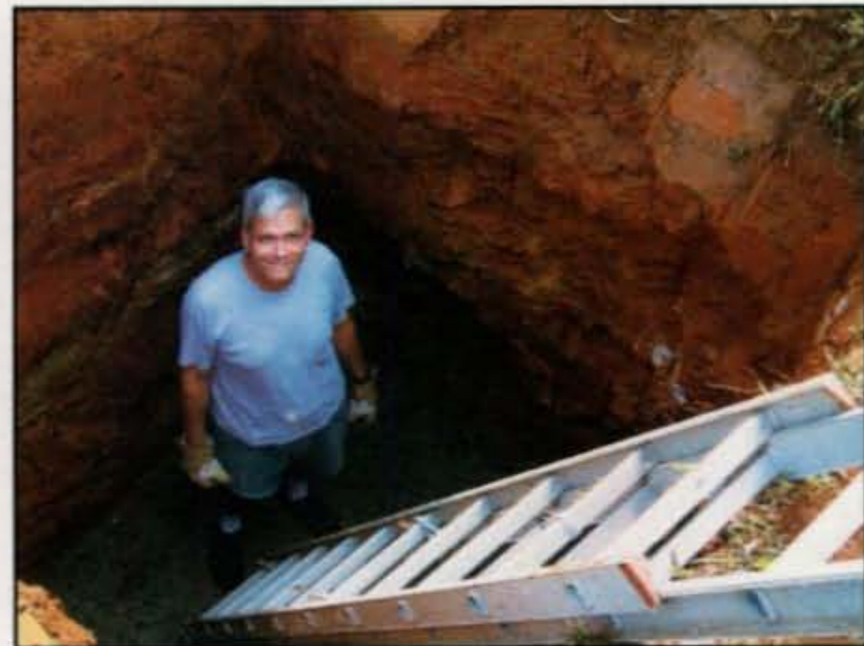
When you move to a new QTH you have to get the antennas up, right? Tom, N4XP, had to put in a substantial concrete base for his new 89-foot, motorized crank-up tower. Here he stands in the hole he eventually filled with 12 yards of concrete. (Photo courtesy of Tim, N4XP)
