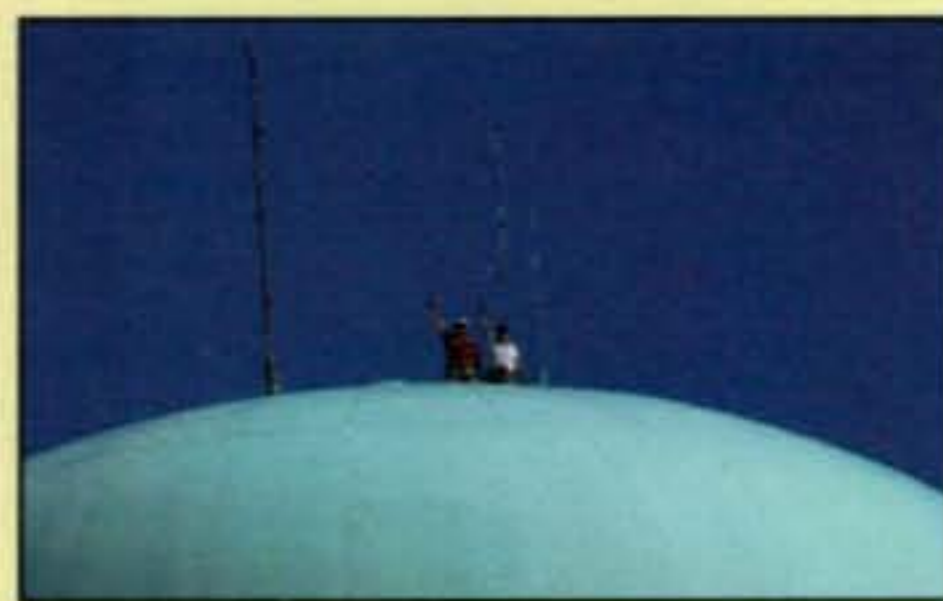
Larry Cole, N4IWP, and Marty Williamson, KB4ZUN, complete the repeater antenna installation in Georgia.
