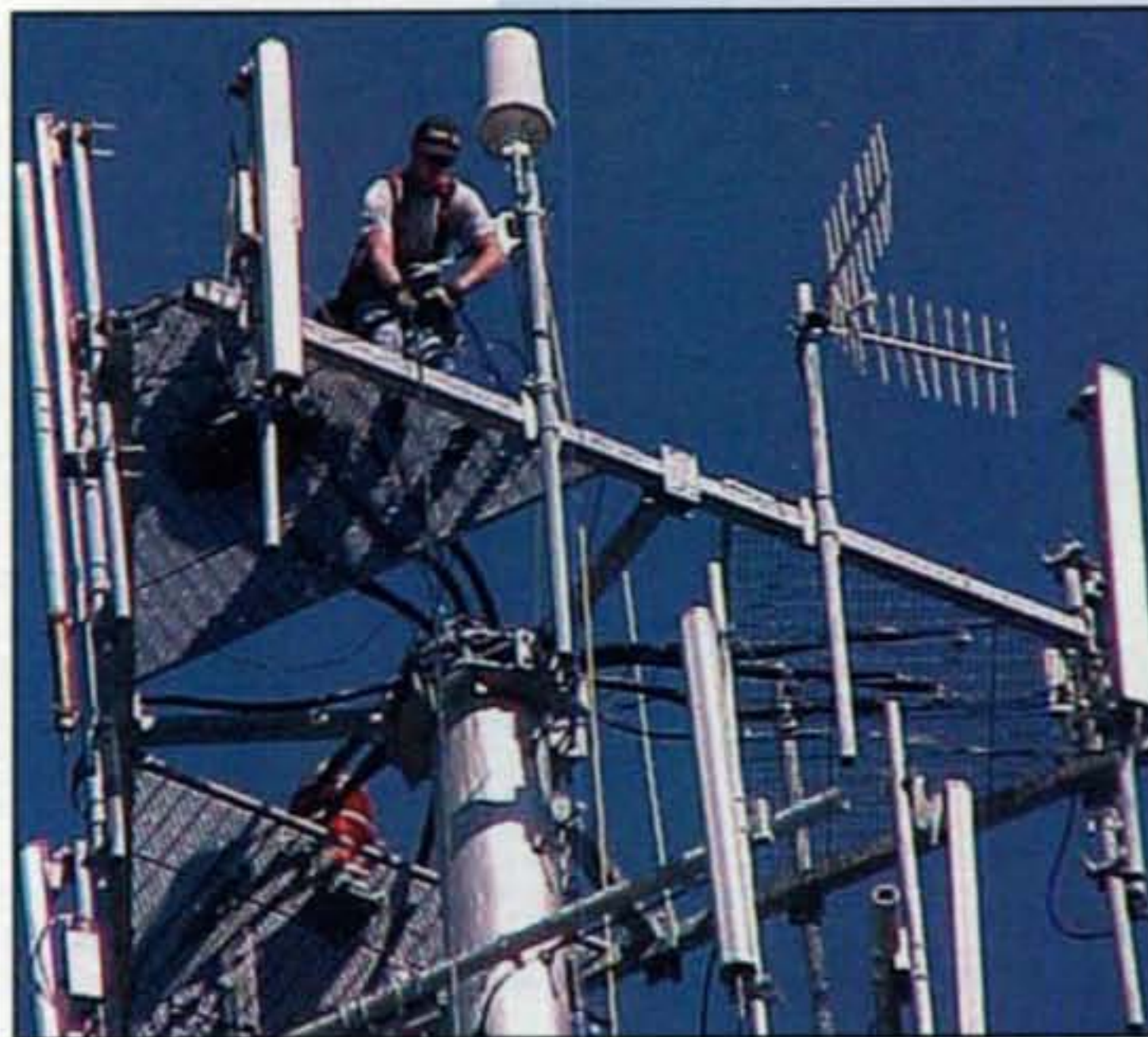
A SkyExtender installed at the top of a tower. The SkyExtender is the white tube near the tower worker's head. Its relatively compact size, simple interface requirements (Ethernet UTP for power and data), and relatively high power (44.5 dBi) using unlicensed 802.11a spectrum and equipment (with proprietary software and protocols) make it an attractive alternative to Cable and DSL for internet access. (Photo courtesy SkyPilot Network Inc.)
