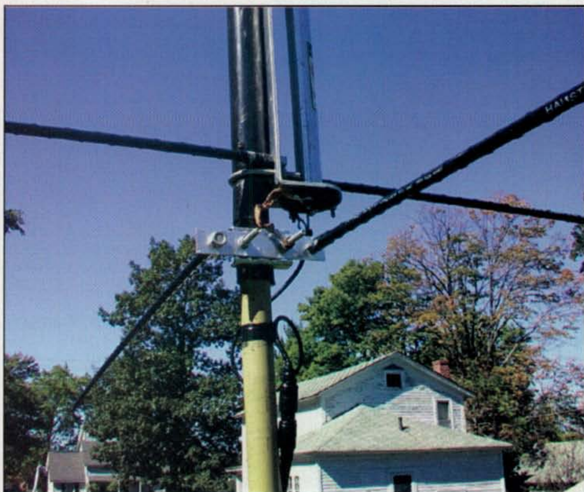
Photo C— The antenna base, showing feedline connection and other details.
