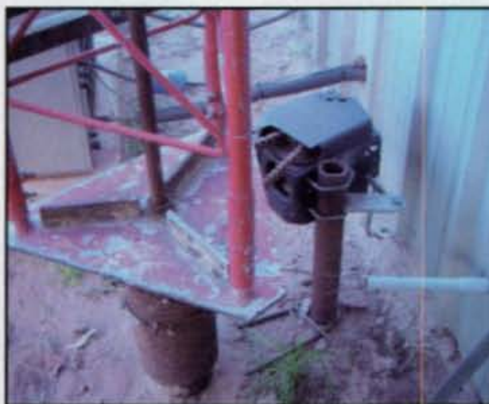
The unique tower rotator, which is a truck winch linked to the tower by a chain. The cable entering and exiting the short piece of PVC pipe is tied to the direction indicator that is part of the maps on the wall inside the shack.
