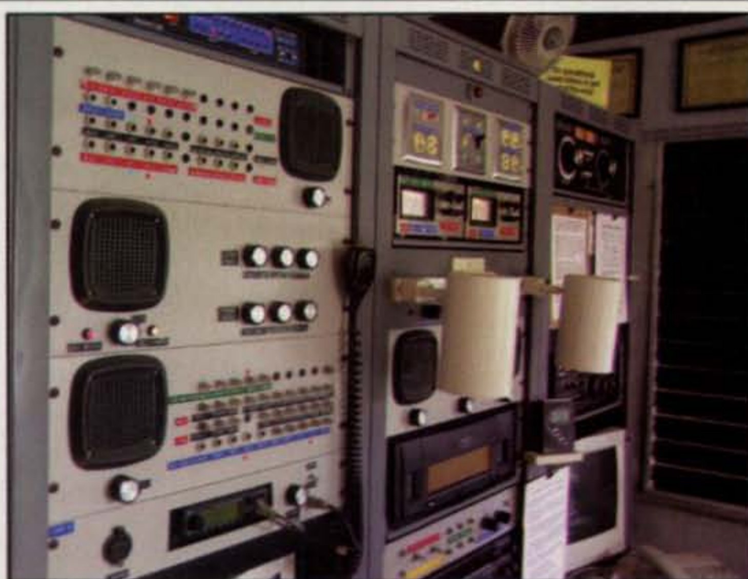
Photo E– Custom-built segments include patch panels, line amplifier, phone patch, and speakers. In addition, the track lighting discussed in the "FAQ" section is visible in the center rack.
