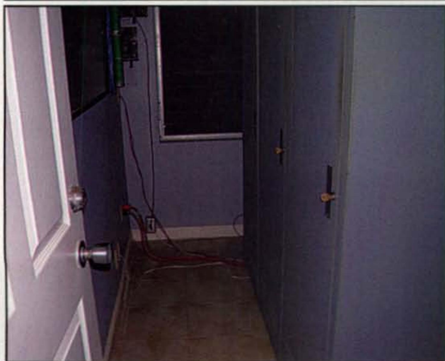
Photo D– Leaving space between the racks and the wall makes it easy to access the service doors at the rear for making changes or doing maintenance or repairs.
