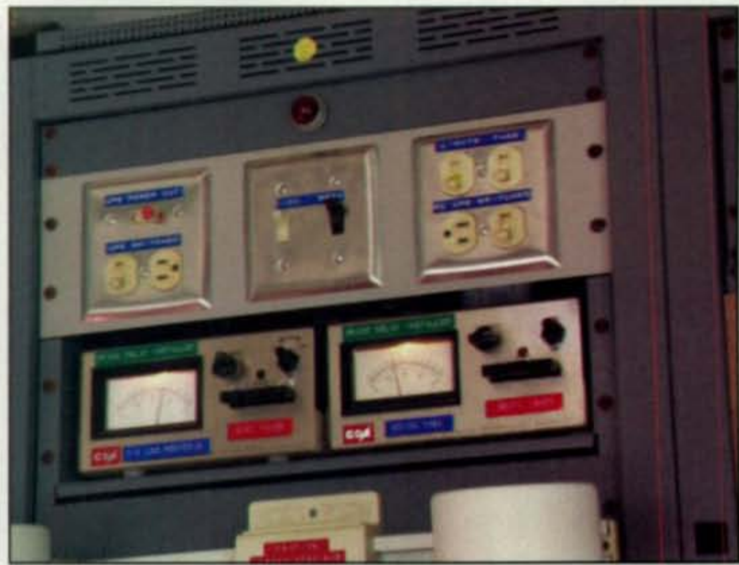
Photo C— All AC power distribution is handled inside the center rack, with various switches easily accessible at the top of the unit.
