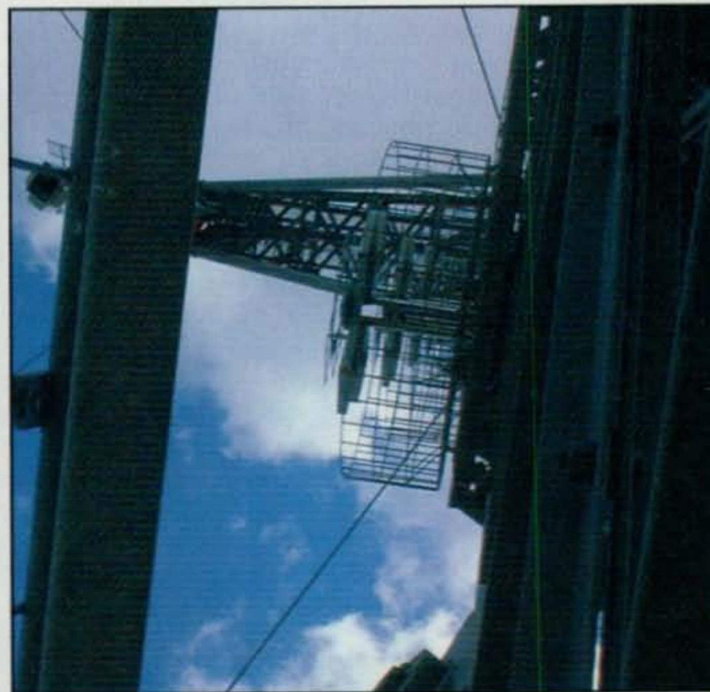
Photo B— A circularly-polarized FM broadcast antenna (center), shot from inside the tower at 1500 feet, looking up toward a horizontal "candelabra" section at 1800 feet.
