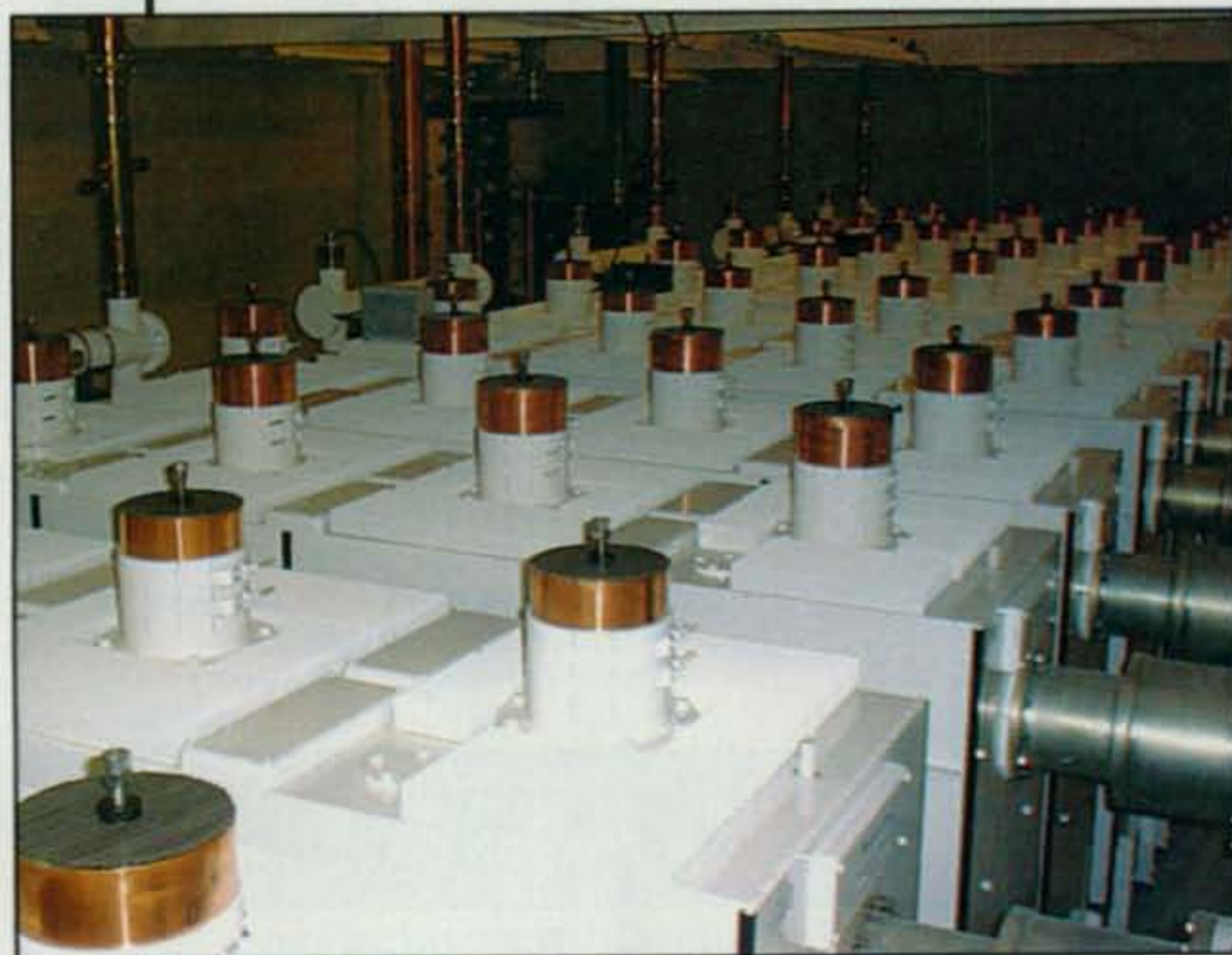
Photo A— Combining eight transmitters on one antenna.
