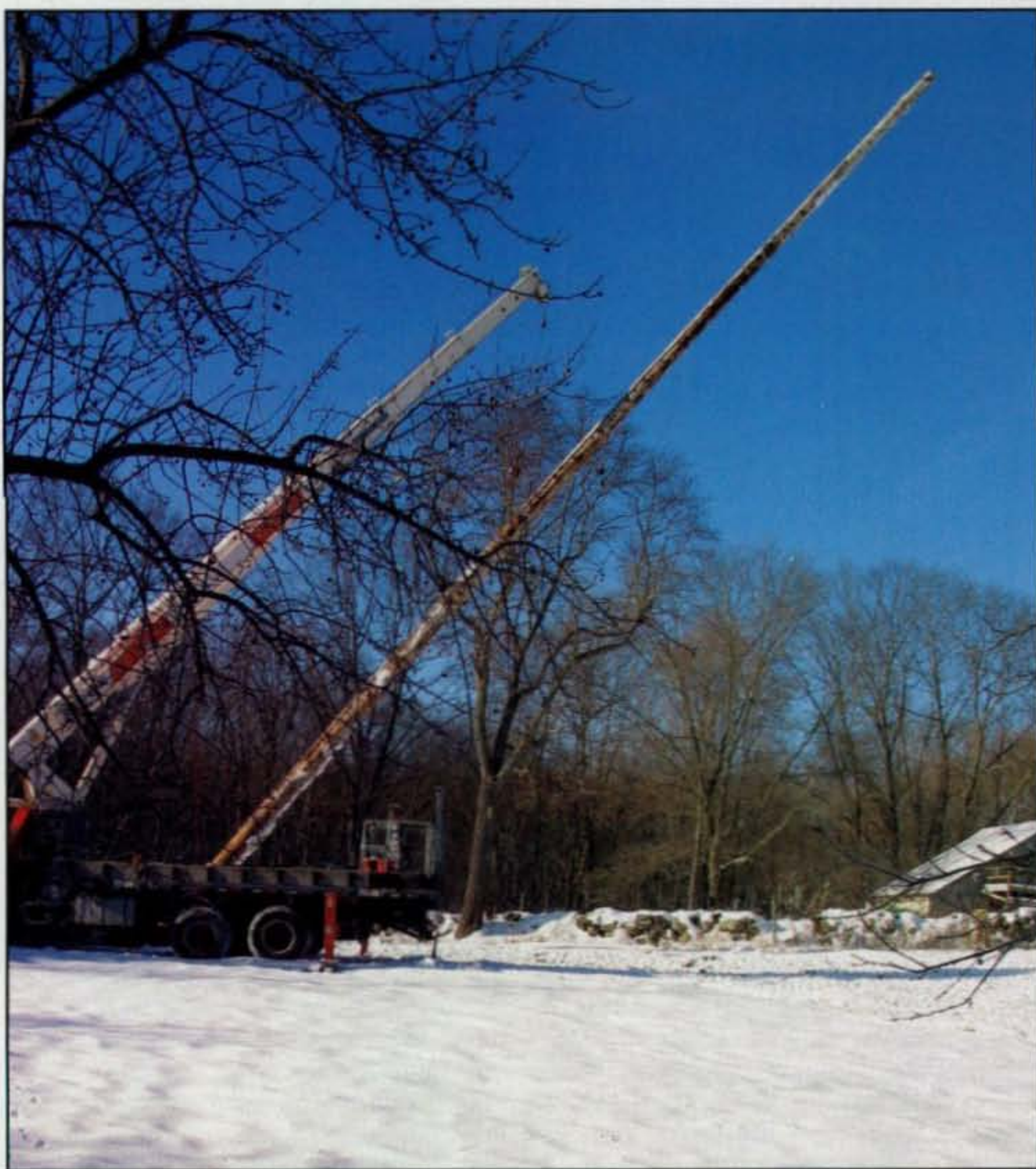
The crane (now out of the mud) lifts the 100-foot pole into position.
