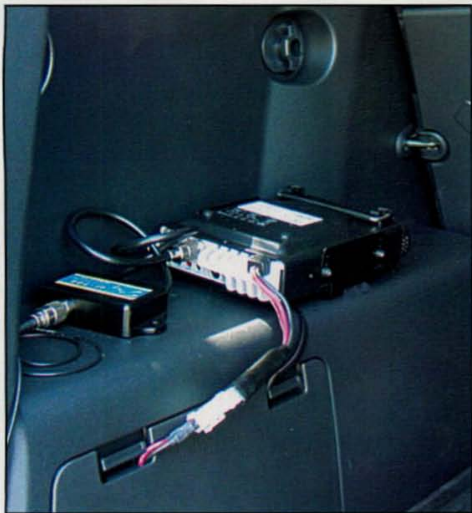
KC1HD mounted the rig in a location where access to cooling air is not an issue. He used beefy 4-gauge wires for power and ground, run directly from the battery (like it says in the textbook!).
