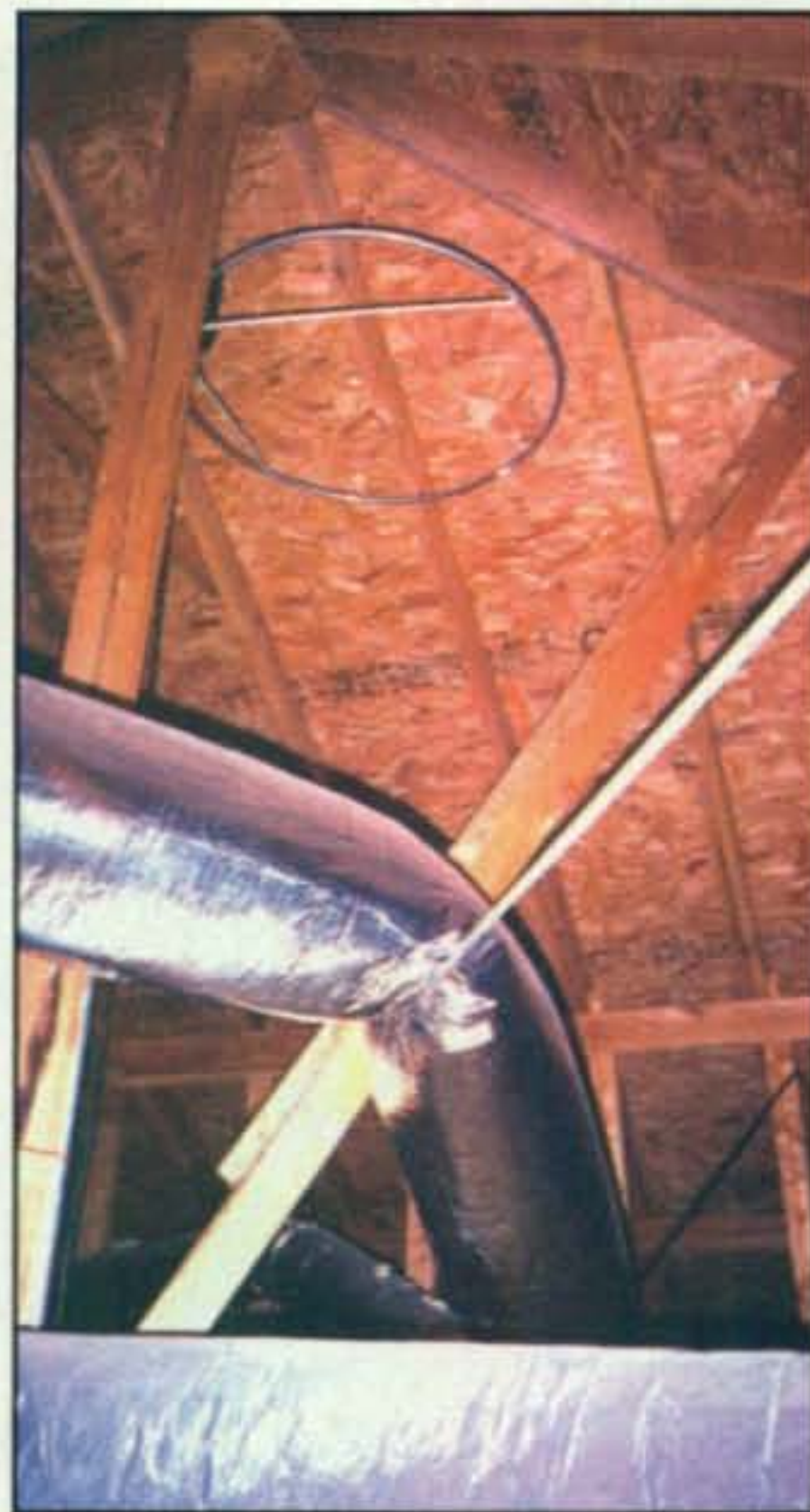
Photo 6— The 6-meter halo and 6-meter/2-meter/70-cm ground plane Don Zelenka, W5AJX installed high in attic of his home. The antennas are approximately 20 feet above ground and have proved their merit by reaching 22 countries plus 270 grid squares. (Photos 6 through 8 courtesy of W5AJX) →
