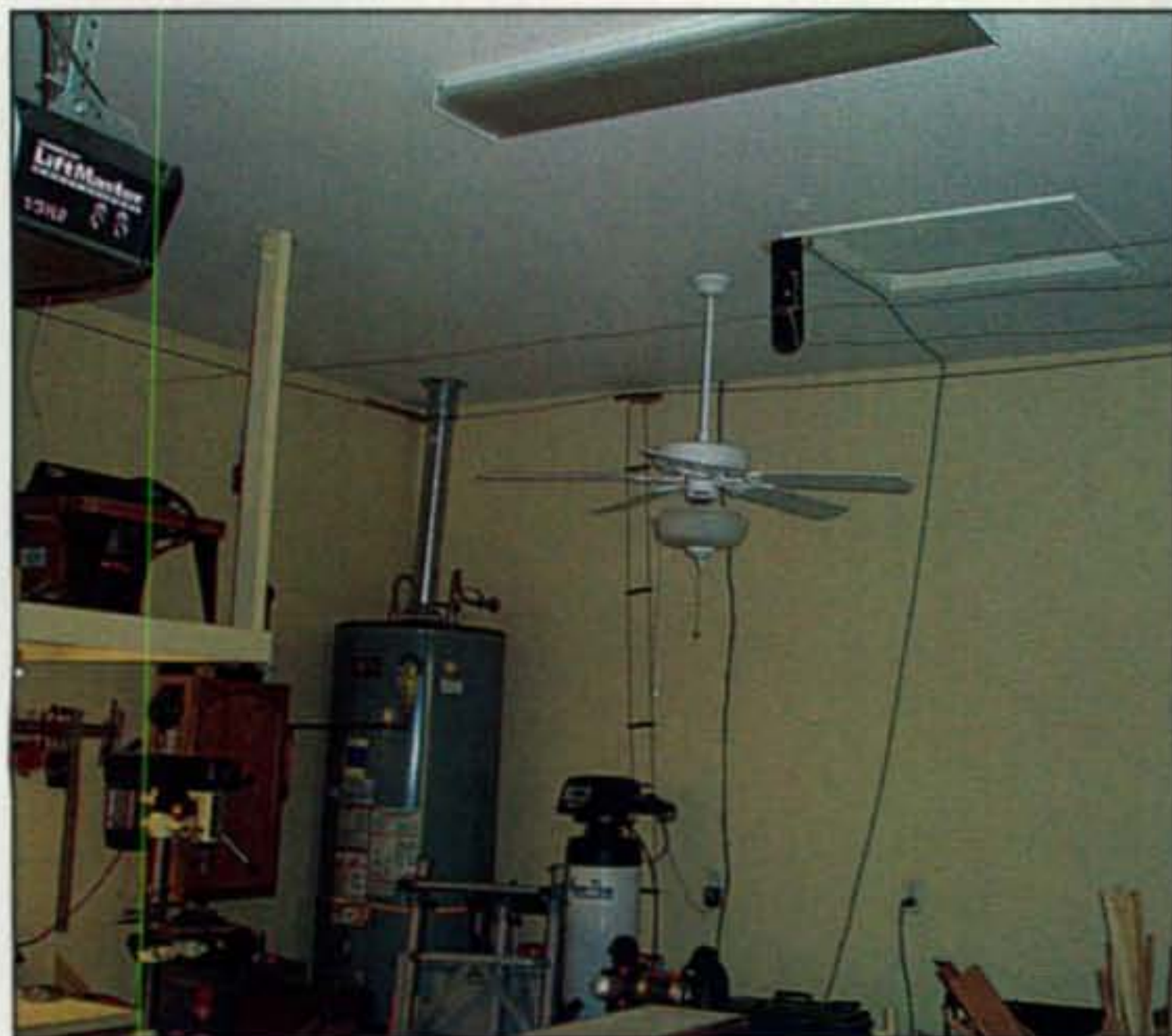
Photo C— An in-garage view of Dave's hidden antennas. The ladder line to right of the water heater goes to a center-fed 40-meter Zepp with its flat-top wires strung around the inside walls of the garage. The two wires on the right side of the ladder line are parts of a homebrew antenna for 20, 15, and 10 meters. The antennas are not over 10 feet above ground, but they do work. (Photo courtesy of AD7JT)
