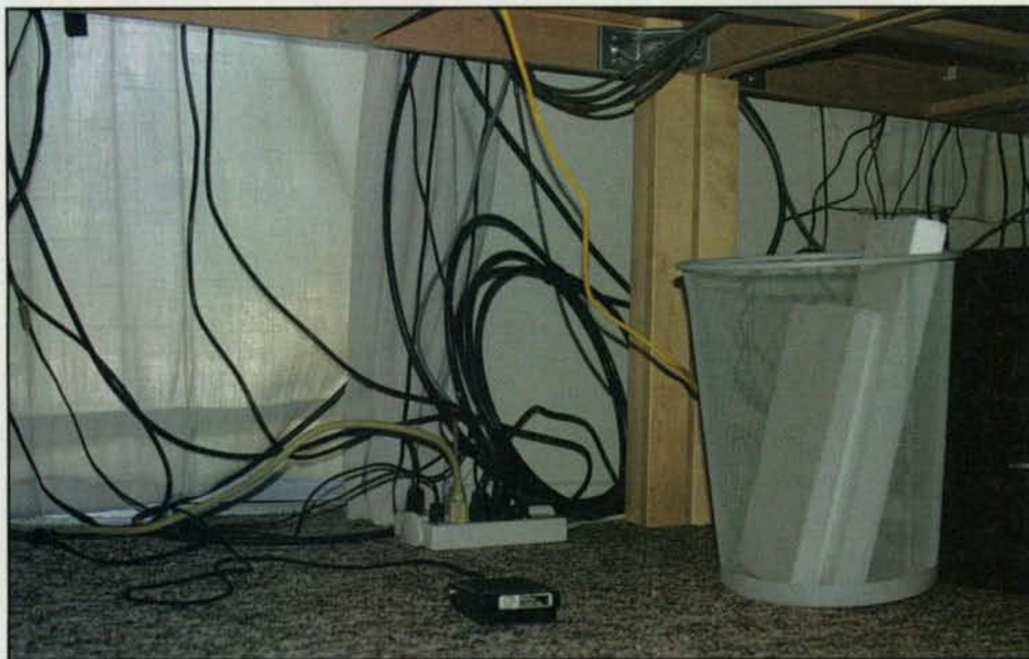
Photo 4— Like many installations, wires on the floor are typical. In this station, these wires will be gathered and nicely bundled with split-plastic wire loom, and trays will be used to hold wires off the floor.
