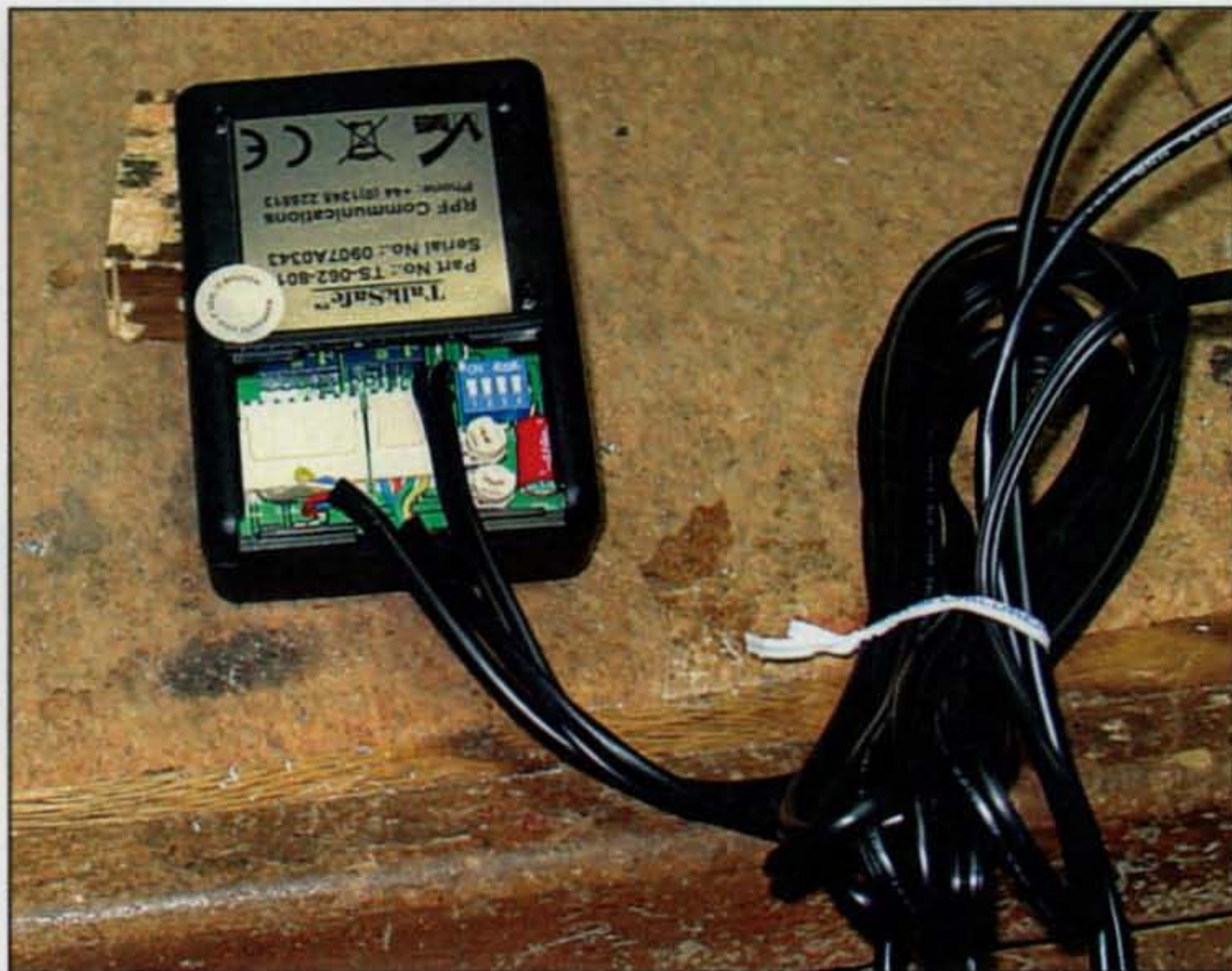
Photo D— Speaker, power, and mic cables plugged in place.
