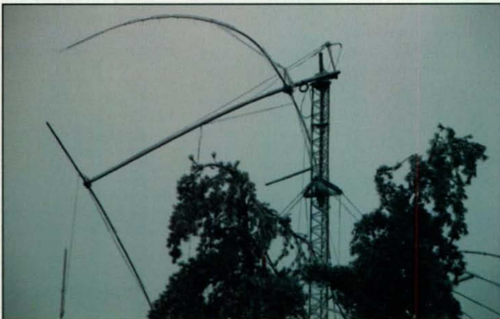
One of the many large antennas at KC1XX's superstation that was destroyed by the storm. (Photo via KC1XX)
