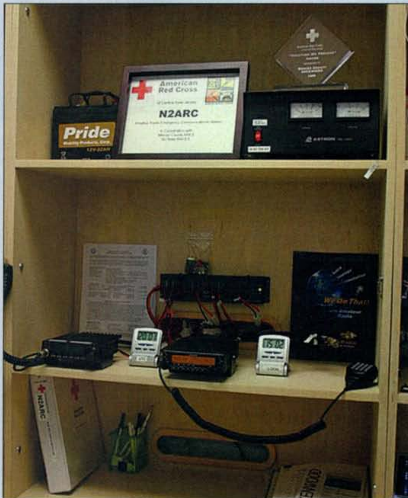
Here is part of the new communications center built by members of the Mercer County ARES/RACES. This unit houses the Alinco DR-235T 220-MHz rig, a Kenwood TM-V71A dual-band radio, and the power distribution system. Other units house HF gear, APRS, and Red Cross radio. (Photo courtesy N2GJ)
