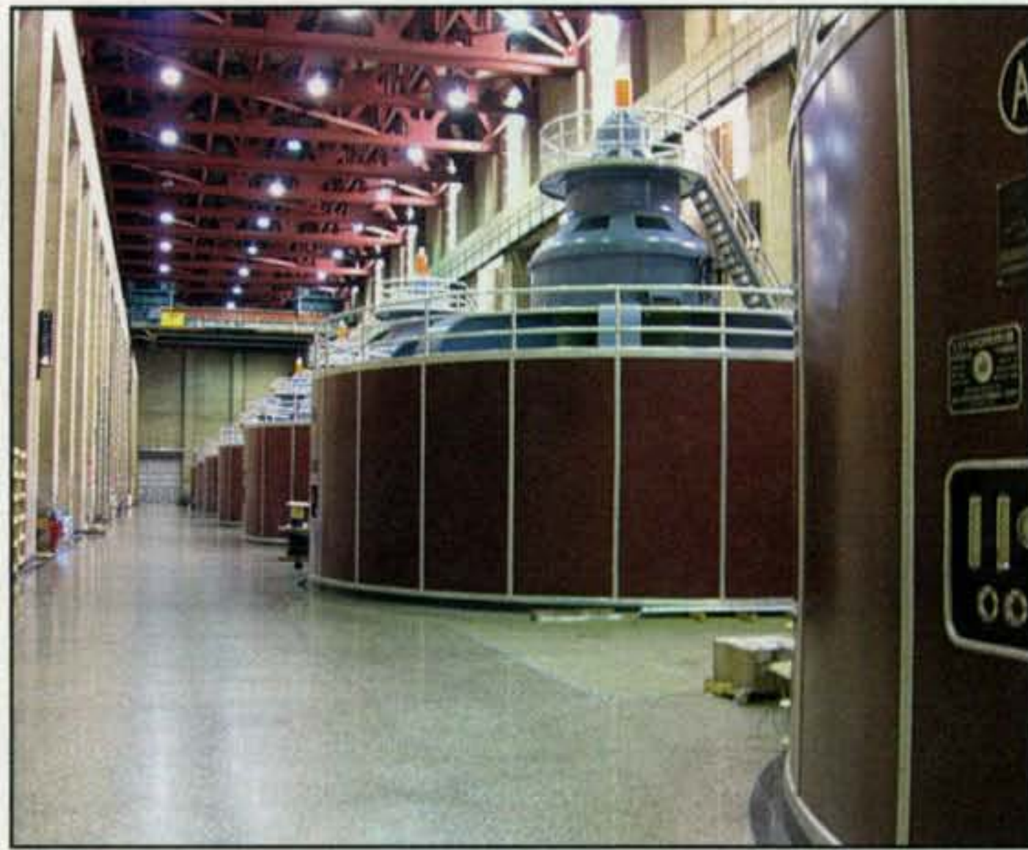
The generator gallery looks as though it was constructed last year, not some seven decades ago. The generators churn out their power without a fuss, practically vibration free.
