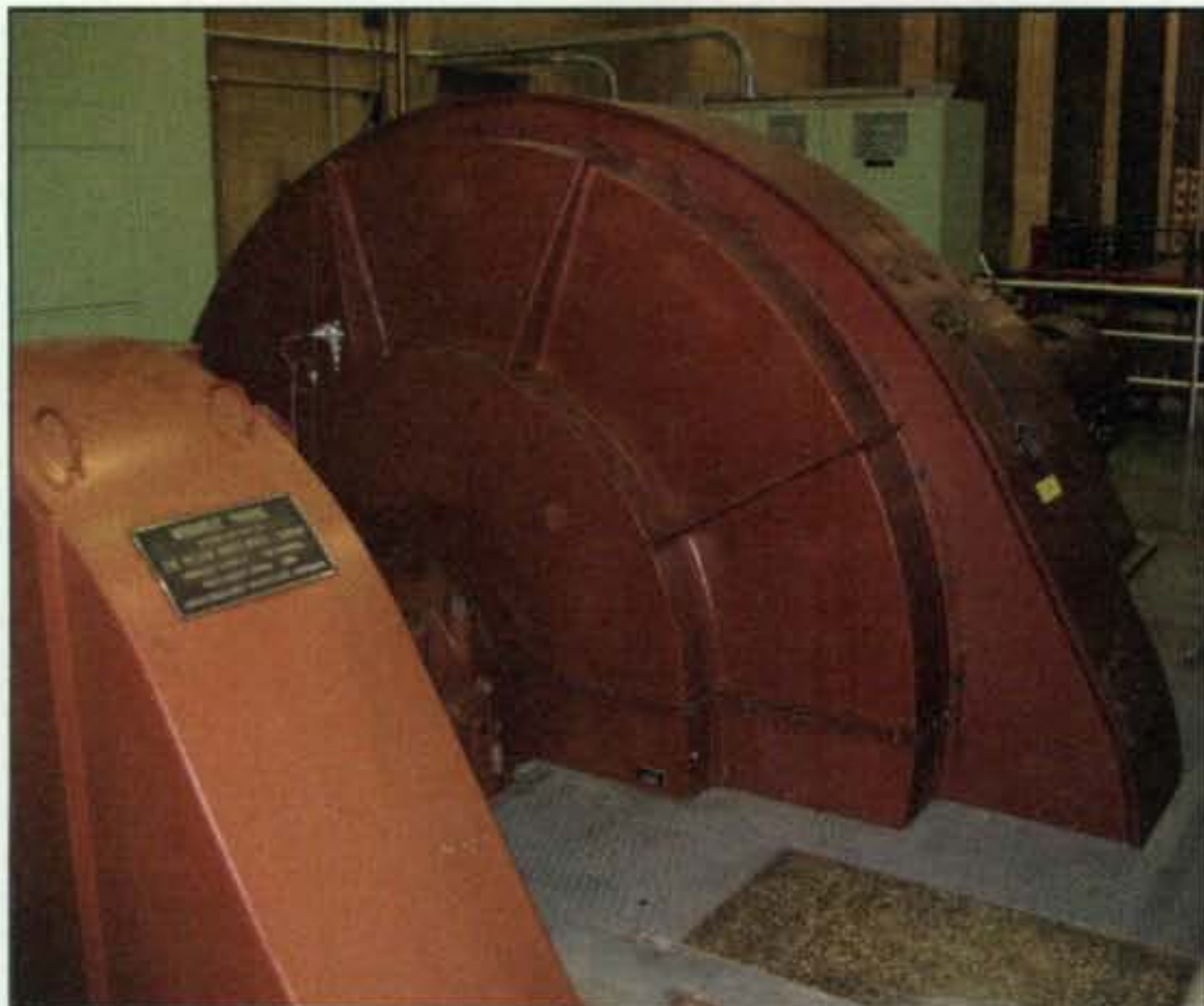
The first generator viewed by the author at Hoover Dam—a “small” 3500 hp water-wheel-driven unit that provides power for dam operations.
