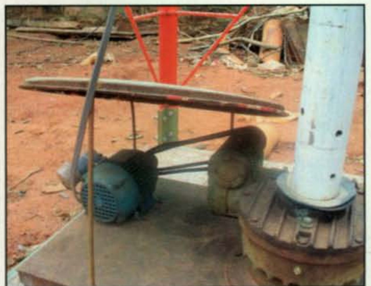
To turn the antenna Doug had this installed—a rotating mast running from the tower base all the way to the top. The mast is turned by the motor and gear box mounted at the base. (Photo courtesy of ZP6CW)
