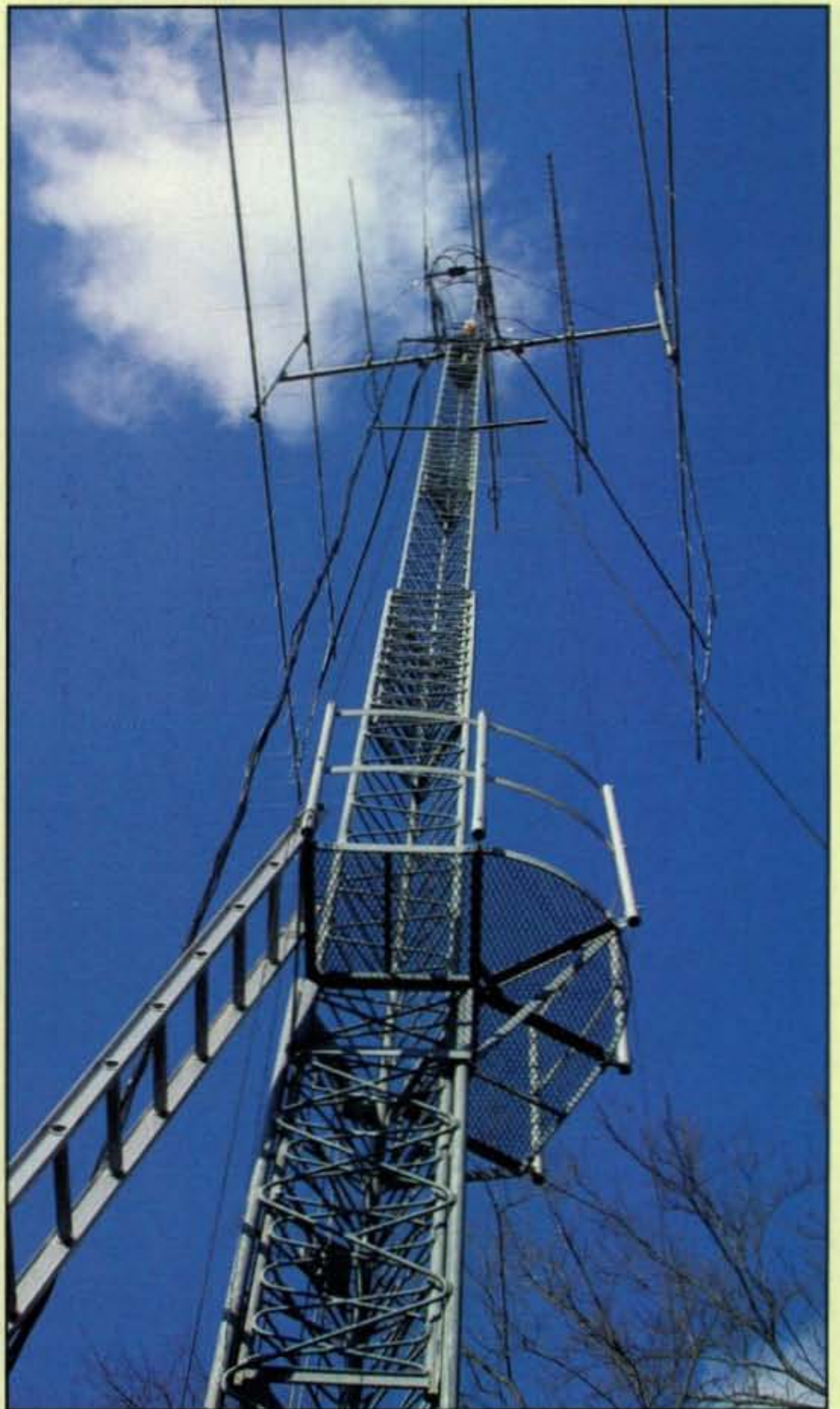
A work platform has been built at the 20-foot level of Joe's tower, allowing him to crank down the antennas to work on them without removing them from the tower or needing to climb to the top.
