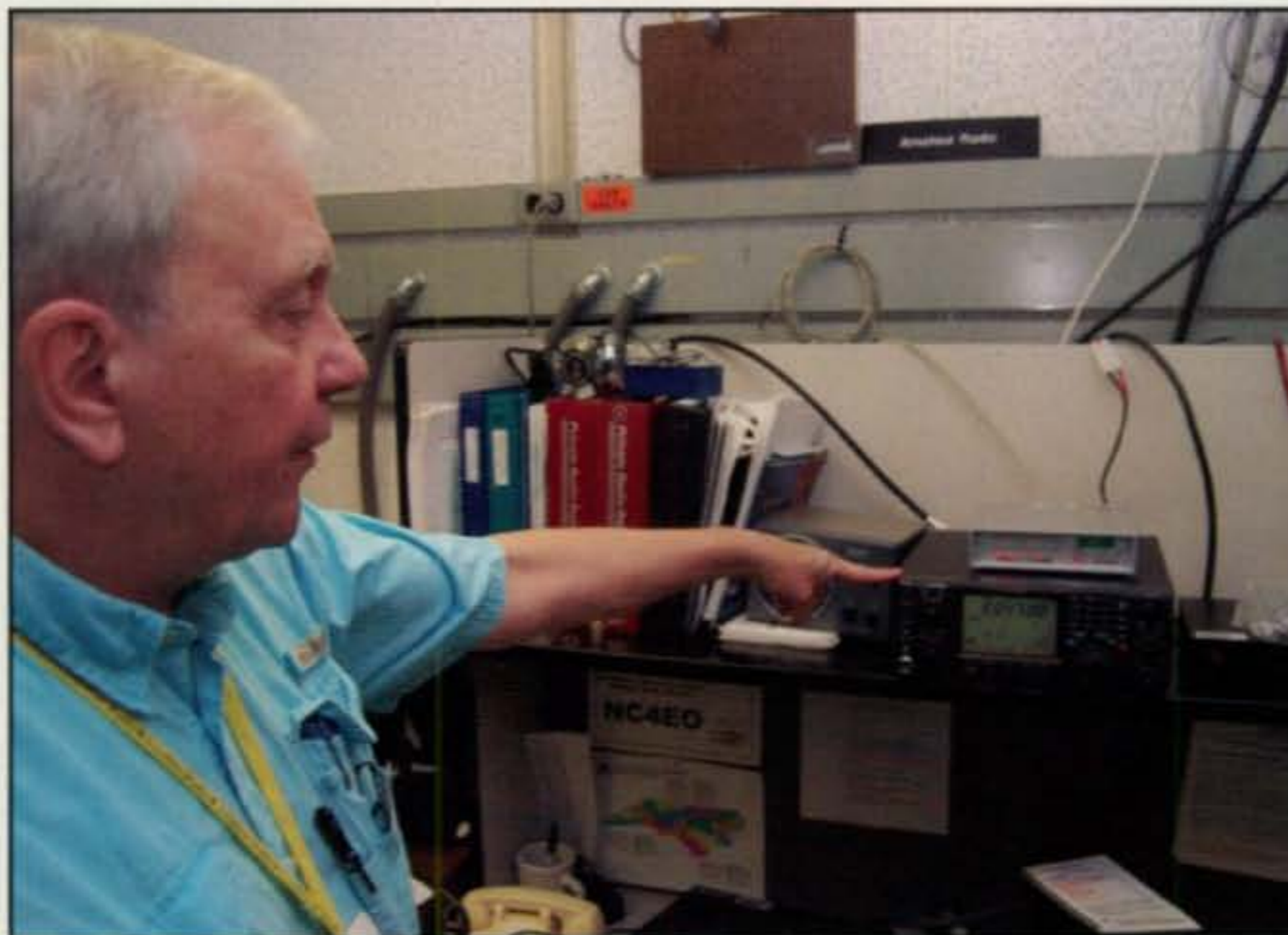
Tom Brown, N4TAB, shows Winlink equipment installed at the North Carolina Emergency Operations Center. (Courtesy of the North Carolina Division of Emergency Management and N4TAB)
