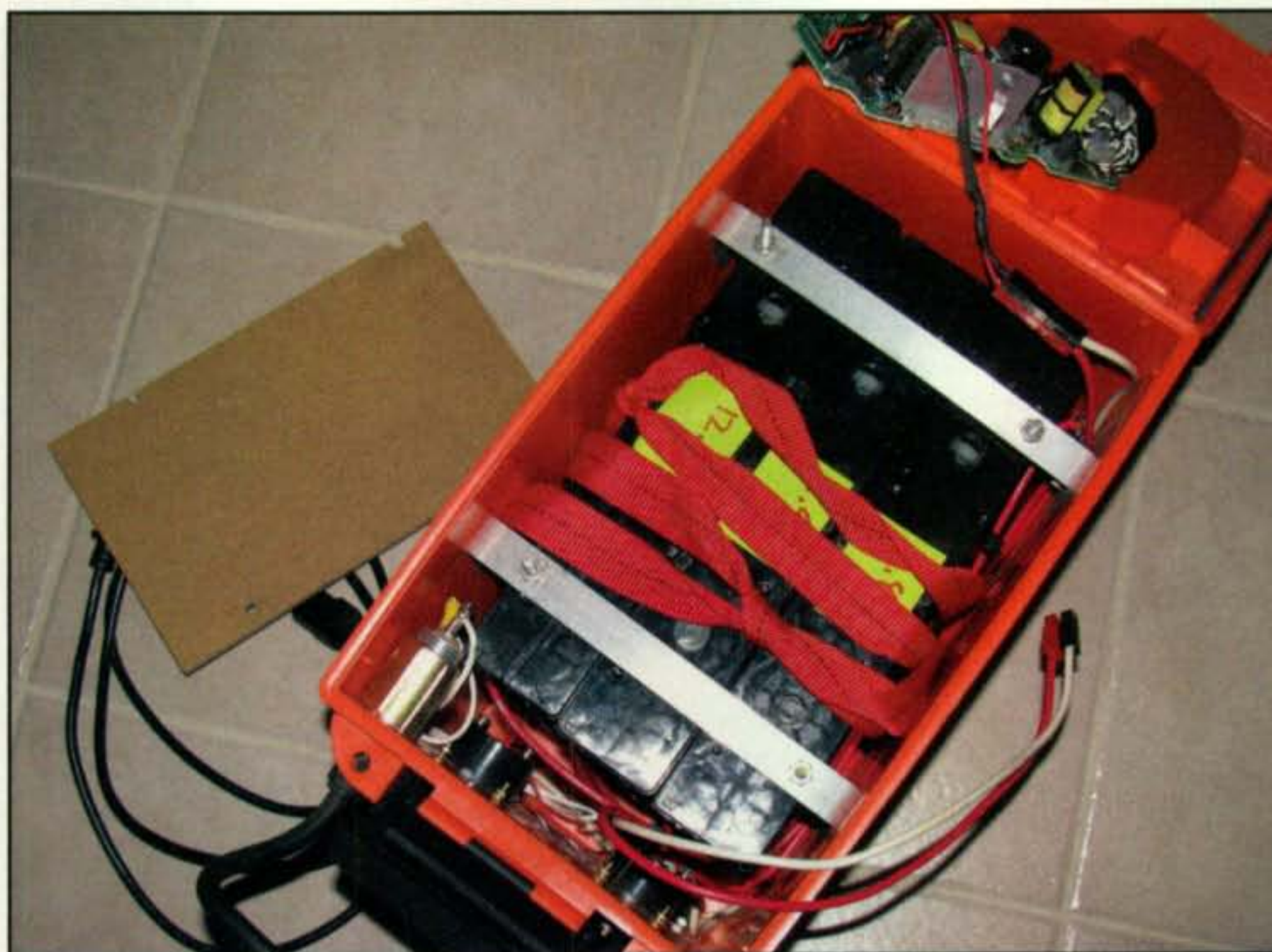
Photo F— Big gel-cells are strapped inside the box. A piece of nylon webbing wrapped around and under the batteries helps to make battery removal easier. A battery charger is included inside the power box.
