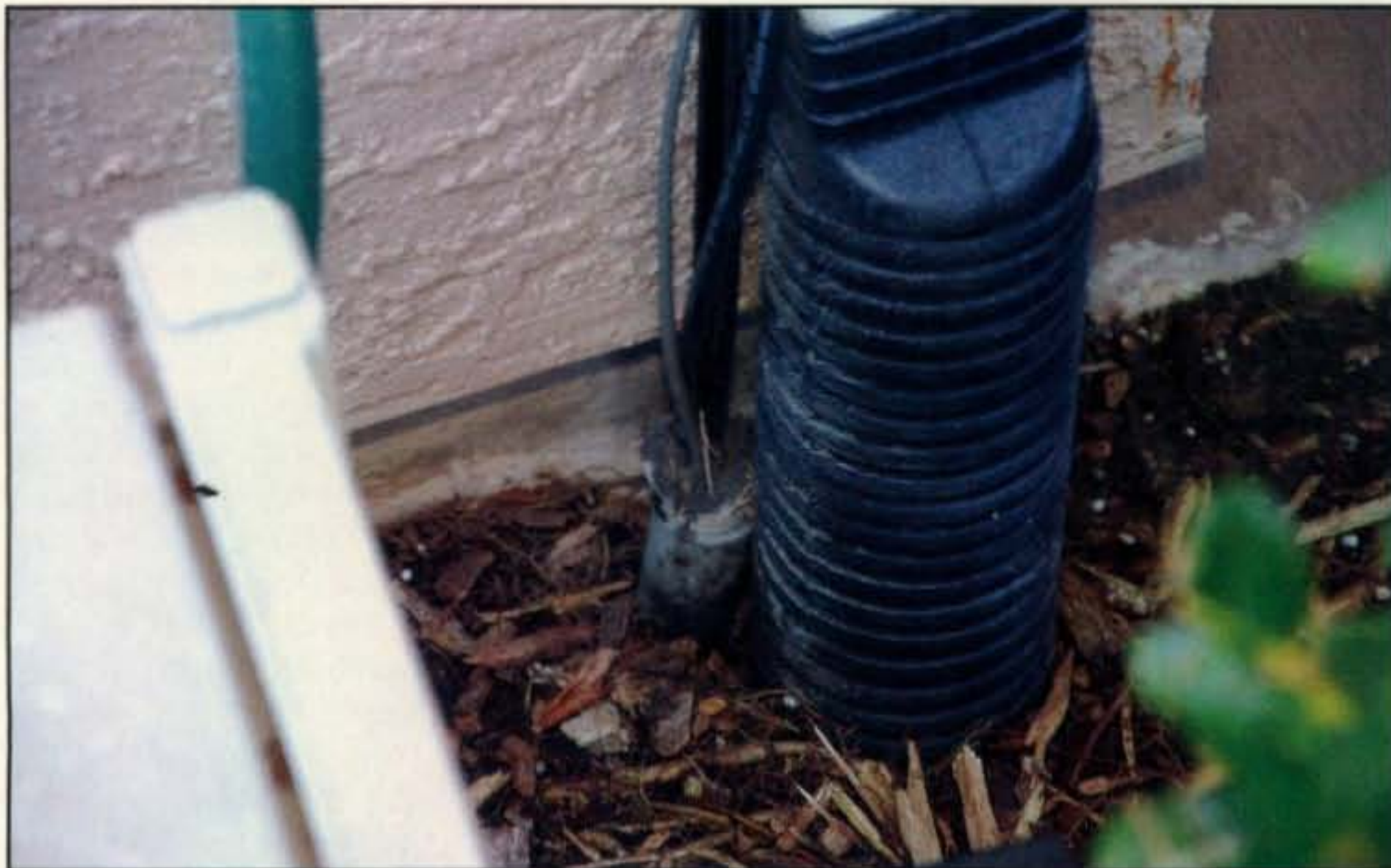
Photo H— Coaxial cables emerging from the ground at KZ5R discreetly attached to the plastic downspout and routed through the attic to the station inside. (Photo courtesy of KZ5R)
