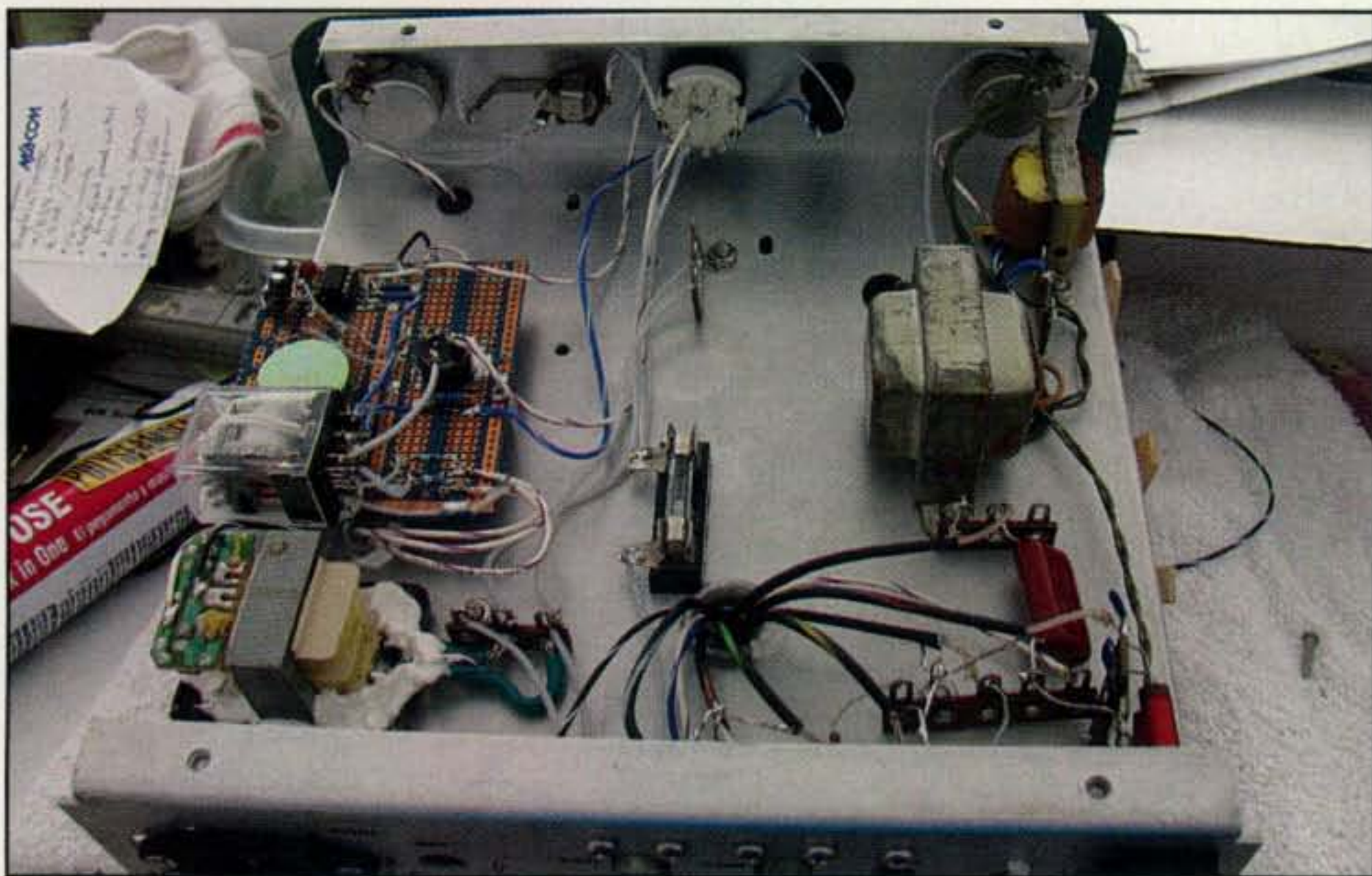
Photo 12 — Oddly, the AC line fuse was missing from the unit. I added a 3AG holder and put a 1/2-amp fuse in there to protect the wall wart, the clock, and the power transformer. Anything continuously plugged into a wall outlet should have some sort of short-circuit protection!
