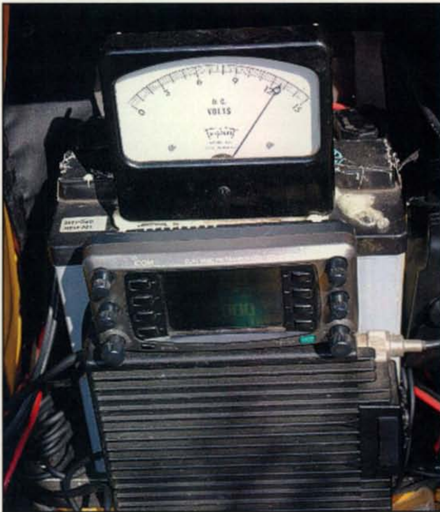
Photo E— A dual-band FM radio is mounted to the side of the gel-cell battery. Note the control head mounted separately and facing out for ease of use, and the voltmeter monitoring the battery's output. The battery in this photo is a 40-amp-hour gel-cell, good for operating HF, but bad on the back if you need to backpack into your operating location.
