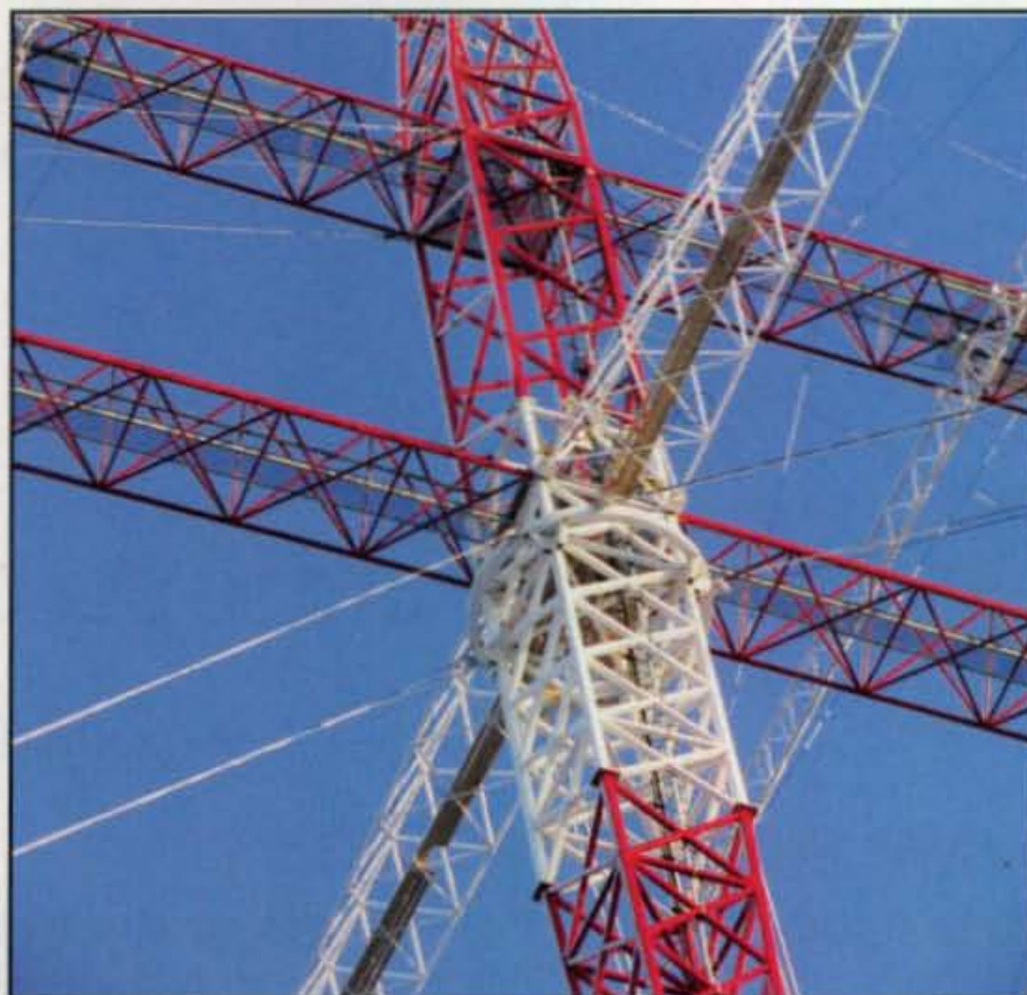
Photo B— A major milestone in the project was when a local steel factory began to make the steel parts of the antenna array. It took six months. The total weight of the steel parts of the antenna array was 39 tons (80,000 lb.) and it took 600 liters (120 gallons) of paint for the tower and elements. Transporting the 12-meter (40-foot) long parts took seven trucks.
