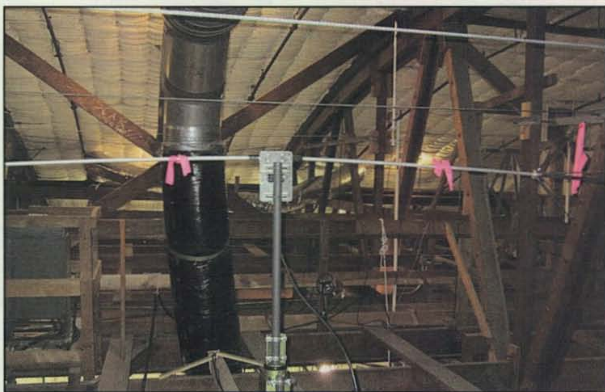
Photo B— The Comet CHV-5X rotatable dipole shares space in the rafters of Studio City Stage 9 with pipes, ducts, and other antenna-unfriendly objects, but it still works! (Photo by John Amodeo, NN6JA)
