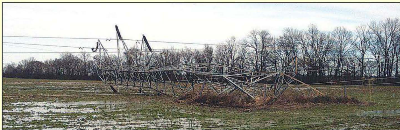
Photo I— A large electrical power line transmission tower lies on its side in Arkansas County after storms ravaged the area. (Courtesy of NWS)
