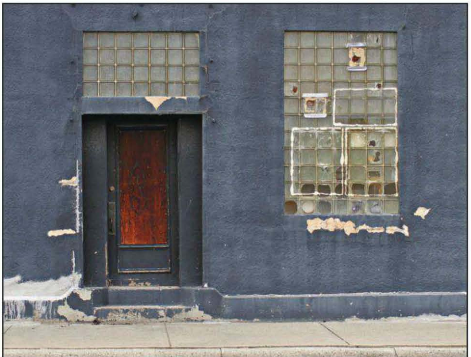
Photo 2– Vanity4Hams' corporate headquarters are designed to minimize overhead expenses, thereby reducing costs to its clients. Damage to the building's façade was the result of a recent exchange of gunfire between corporate personnel and personnel from the Bureau of Alcohol, Tobacco, and Firearms and Explosives (ATF), who were mistaken for rival "businessmen." The building will be repaired this summer. 6
