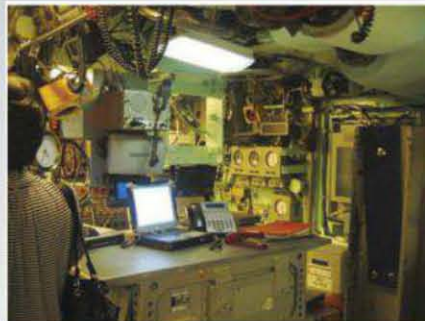
DELTA switches in nuclear sub comm rooms
