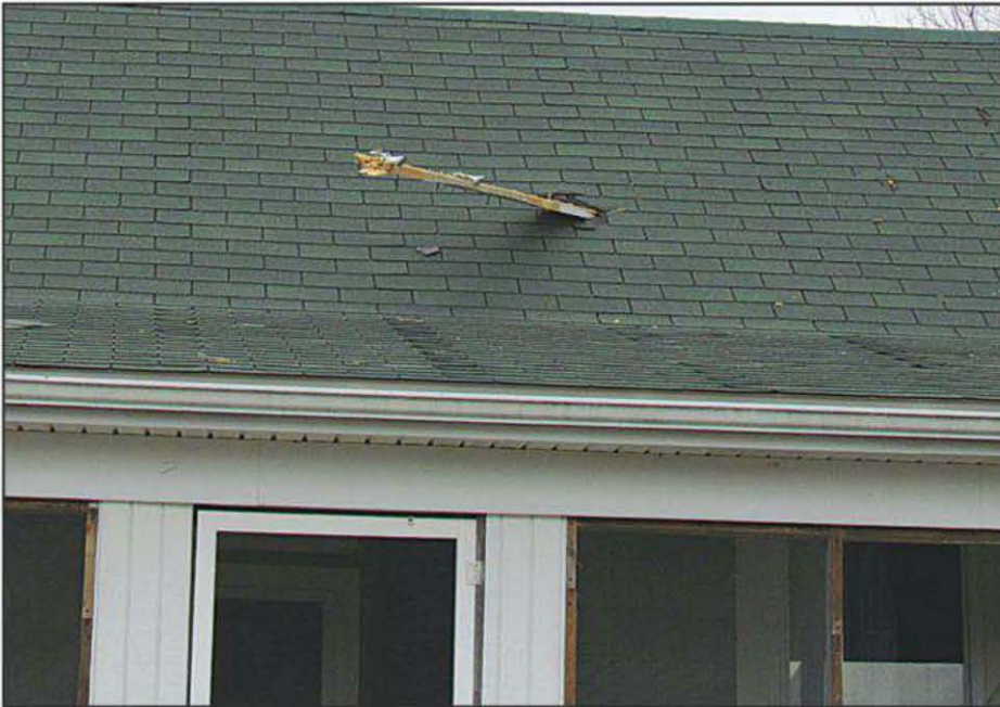
A piece of wood, propelled by tornado-force wind, impaled the roof of this house in Holton, Indiana. (Courtesy of KC9RLC)
