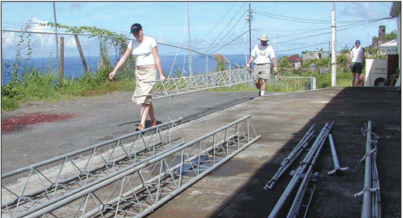
Laura (daughter of Ulf, DL5AXX) and George, N2GA, carrying tower sections into position for assembly.
