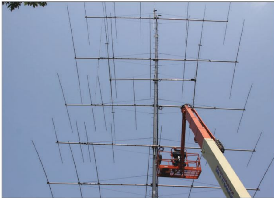
Photo E. Stacked antennas on a 150-foot tower at K4VV can be used by remote operators.
