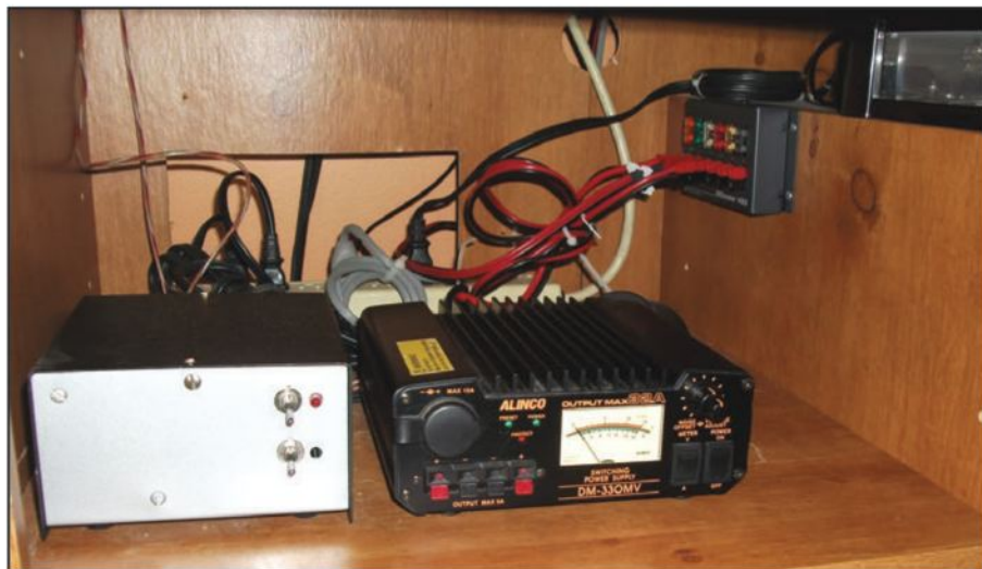
Photo E. The homebrew power supply to the left, the switching power supply in the center, and the power supply distribution panel mounted at right rear.
