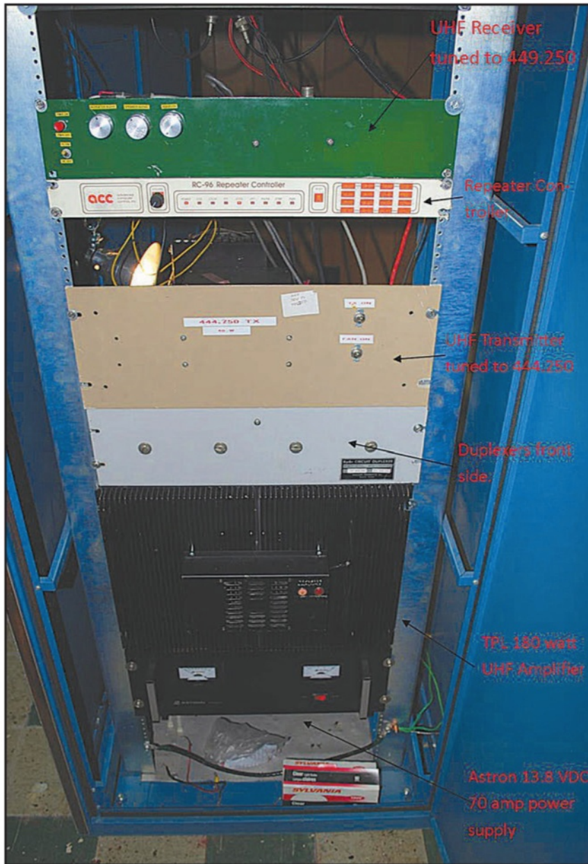
Photo F. The front side of the rack-mounted WS9V repeater system. On the top is the 449.250-MHz receiver and below that are the ACC RC-96 controller, the 444.250 MHz transmitter, the 70-cm BpBr duplexers, the TPL 180 watt amplifier, and the Astron 70 amp 13.8-VDC power supply. Not pictured is the battery backup in case of commercial power failure.
