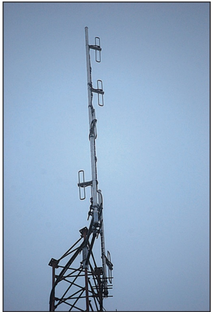
Photo C. An example of a commercial VHF 4-bay (folded-dipole configuration) repeater antenna.
