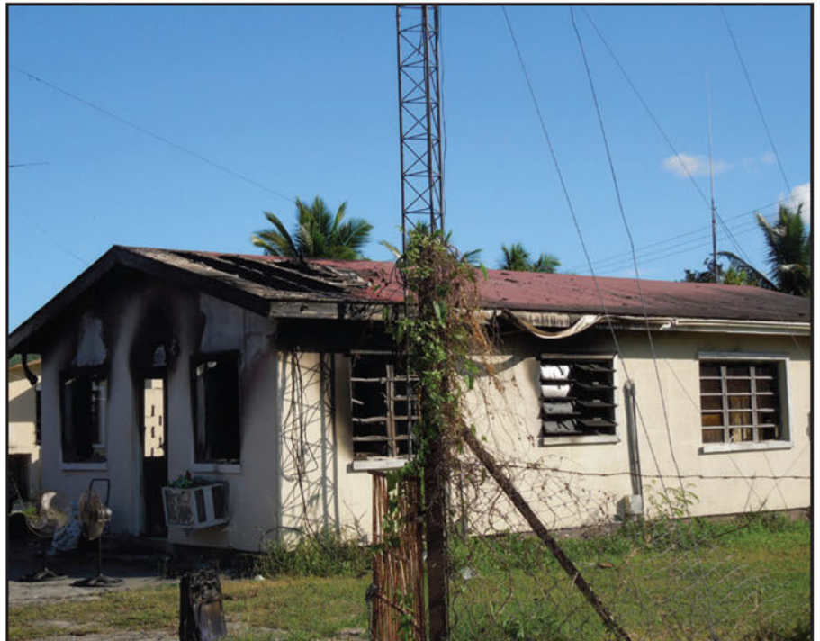
Photo A. V26B shack after the fire. Exterior damage was extensive; interior near total. (Photos courtesy of the author)
