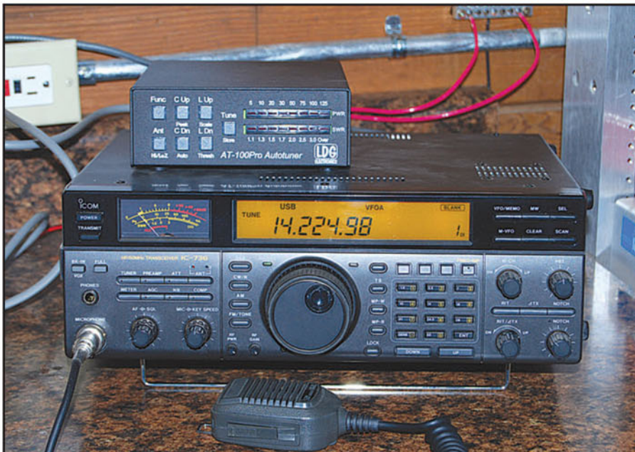
An ICOM transceiver and LDG auto tuner are part of the HF operation at Peaceful Valley Scout Ranch.
