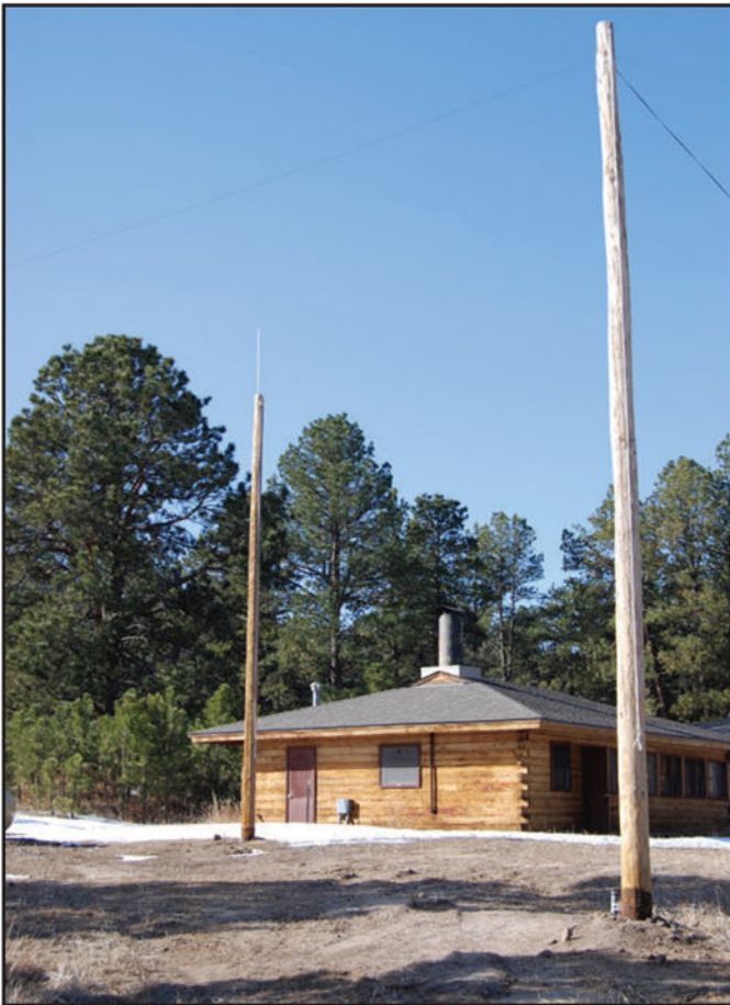
Telephone poles are put to good use in the antenna farm at Peaceful Valley Scout Ranch in Colorado.
