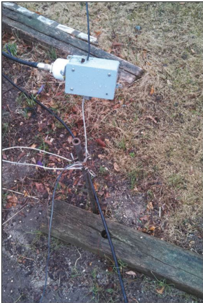
← Photo C. A 220-foot run of LMR-400 feedline connected the station (in photo D) to the antenna, a 125-foot vertical with eight 130-foot radials. (Photo by the author)
