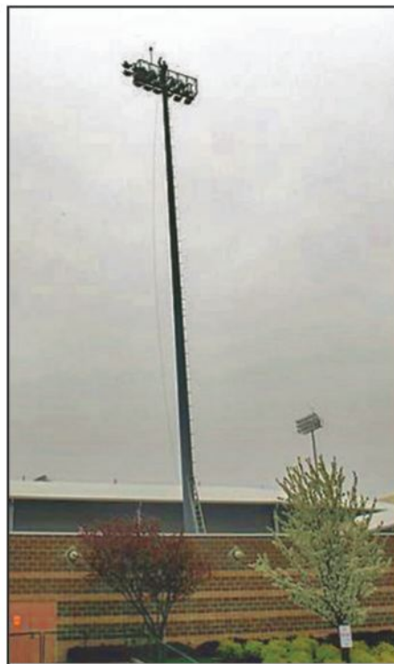
Photo B. Those lights sit atop 130-foot poles ... imagine them as antenna supports (the author did!) (Photo by Mario Nistico)
