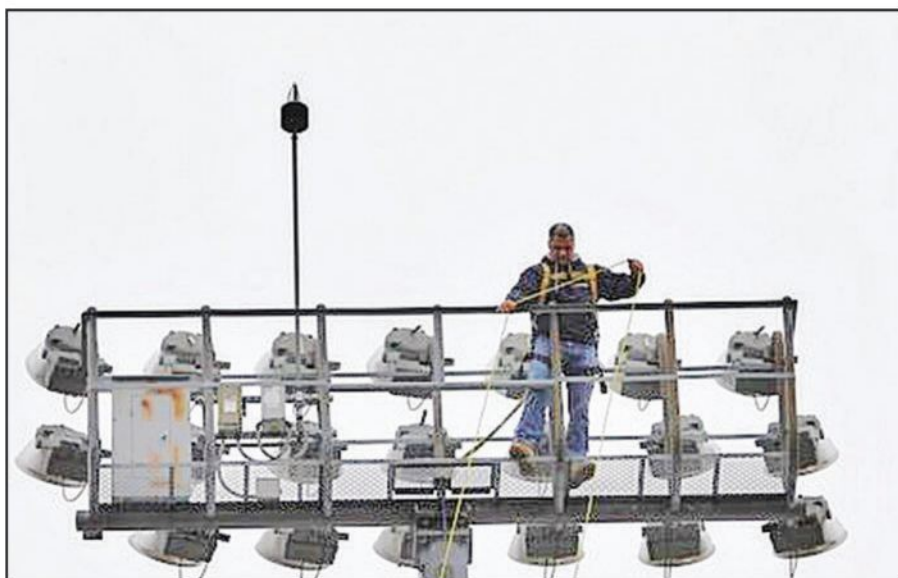
Photo A. The author servicing field lighting at the Long Island Ducks baseball team’s home field in Central Islip, New York. (Photo by Mario Nistico)
