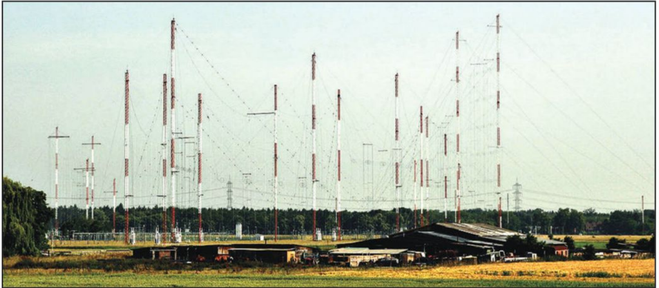
Photo B. This massive Curtain array is used at the Radio Free Europe transmitter site in Biblis, Germany. (Courtesy of Wikipedia)
