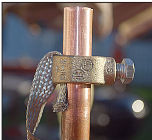
Photo C. Notice that the ground wire braid comes between the clamp and the rod and it is located opposite from the grounding lug.
