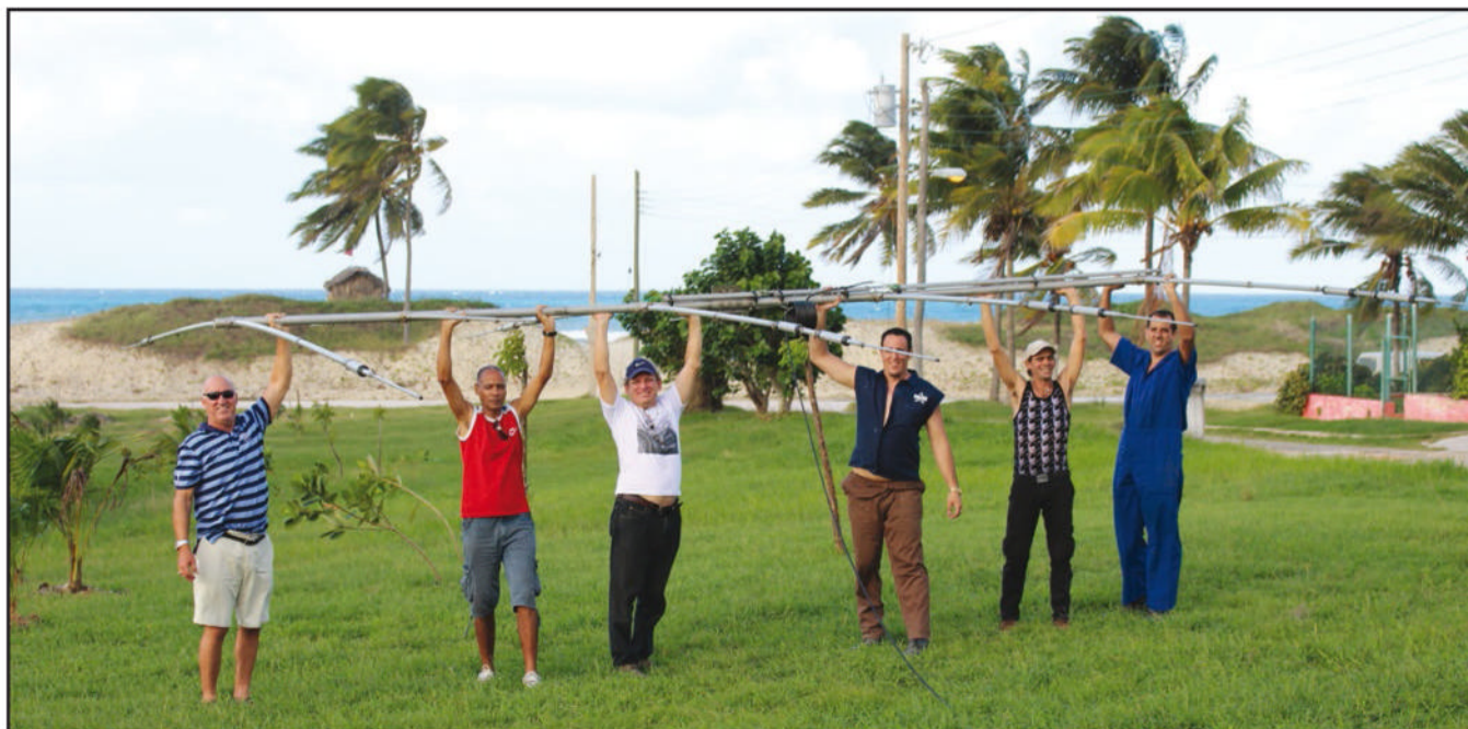
Photo D. The group's 4-element, 6-meter beam held up for tuning prior to installation by, from left, Mark, WC3W; Juan, CM2OY; Roberto, CM2KL; Amed, CO2AME; Alexi, CO2XK; and Michel, CL2TV.
