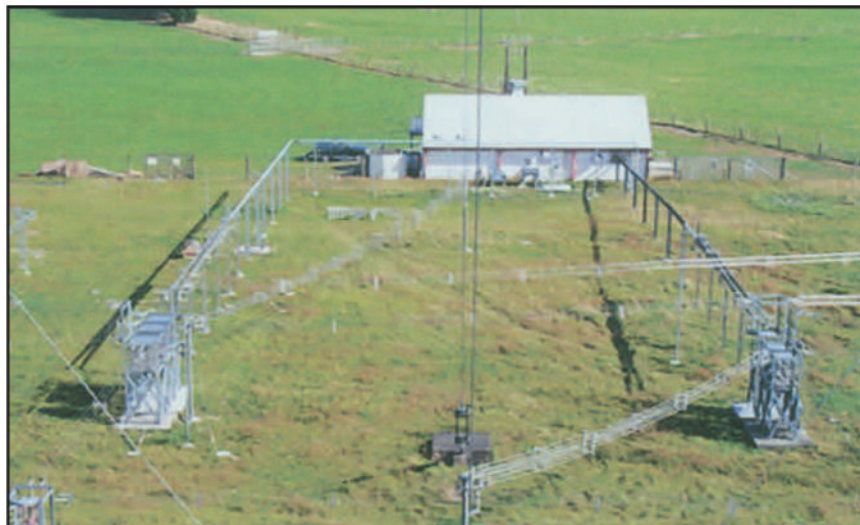
Radio New Zealand's transmitter building at Rangitaiki.
