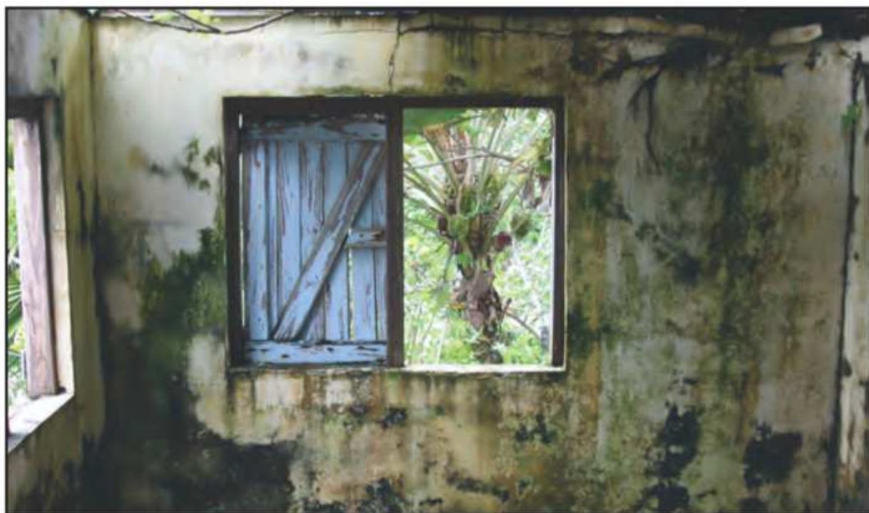
Photo E. Because of constant exposure to the elements, there was mold on all of the interior walls.
