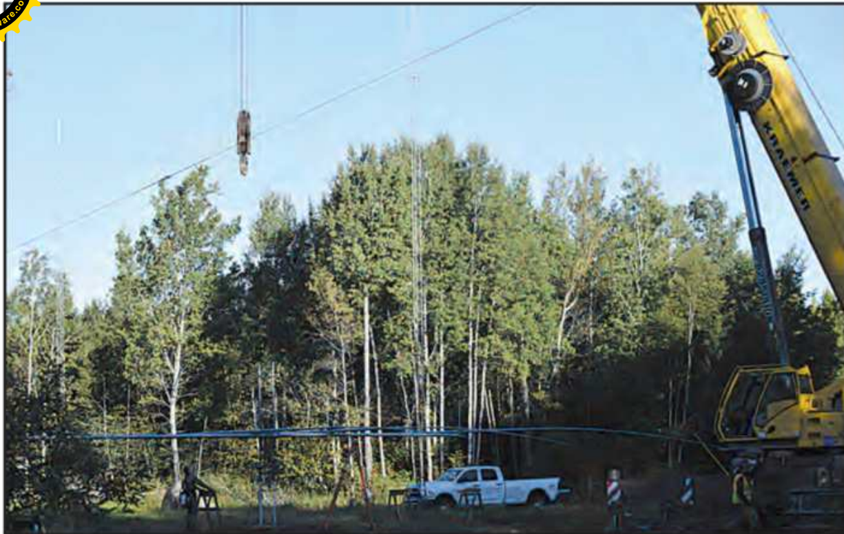
Photo E. In the final stage, the tower is dismantled and ultimately removed by HamEstate.
