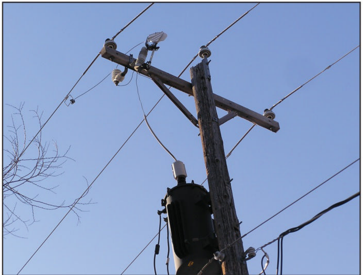
Photo A. Power lines and their support structures can often be the source of interference. In the case that Sherlock investigated, the noise resulted from arcing between a metal crossbrace and loose bolts. (Photos by the author)
