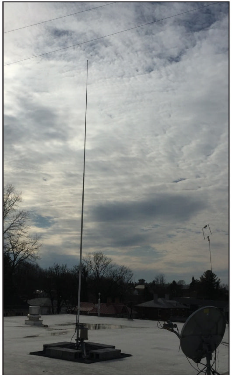
Photo G. Many vertical antennas require antenna tuners.
