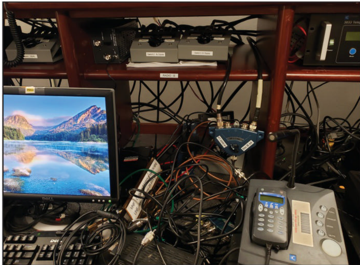
Photo K. Rats' nest of RF cables
