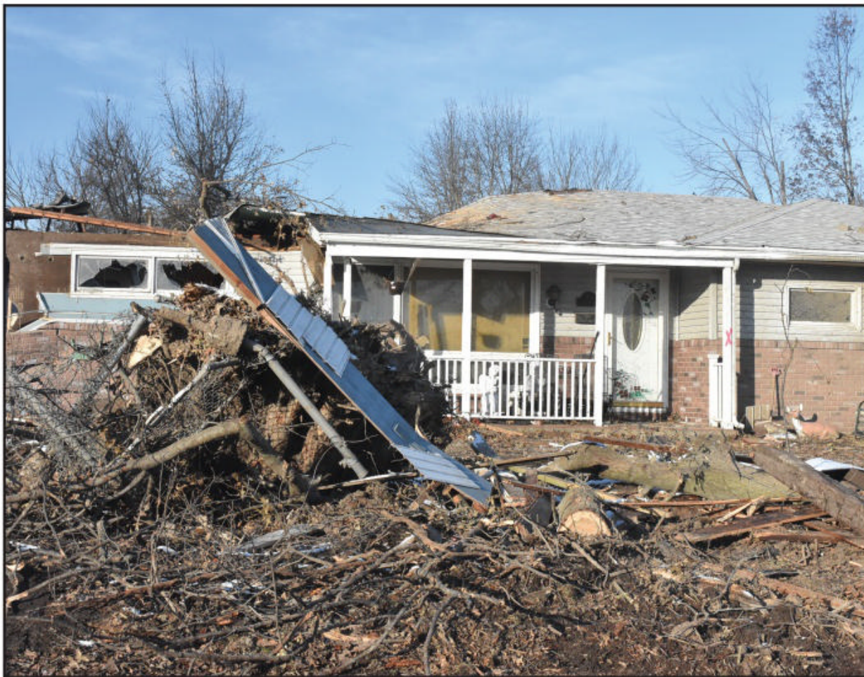
Photo B. One of the many Taylorville homes destroyed by the EF3 tornado.
