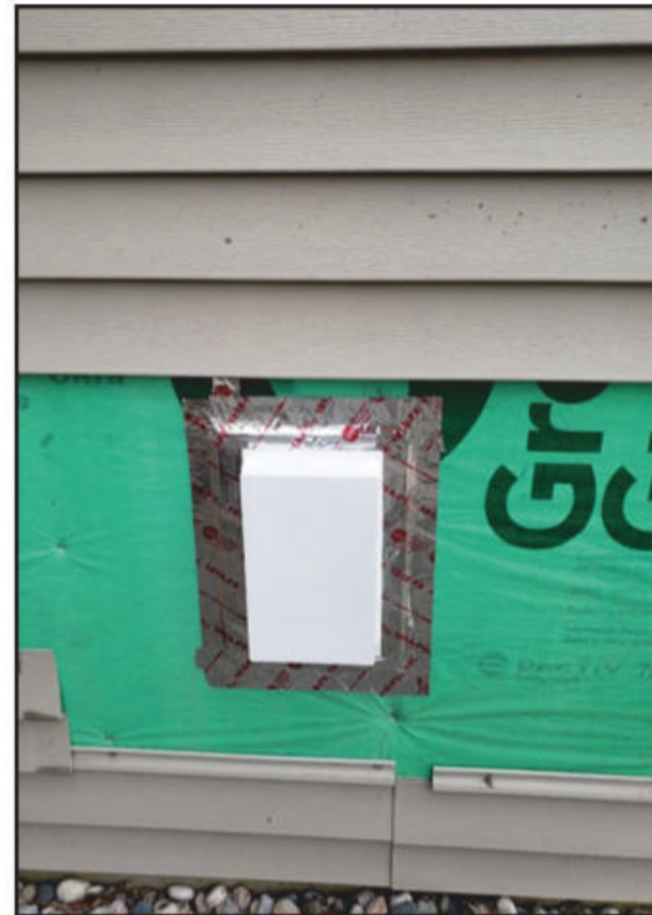
Photo C. Brian's exterior wall. Note the siding removal and placement of the weatherproof enclosure. (Photo by NØBMK)
