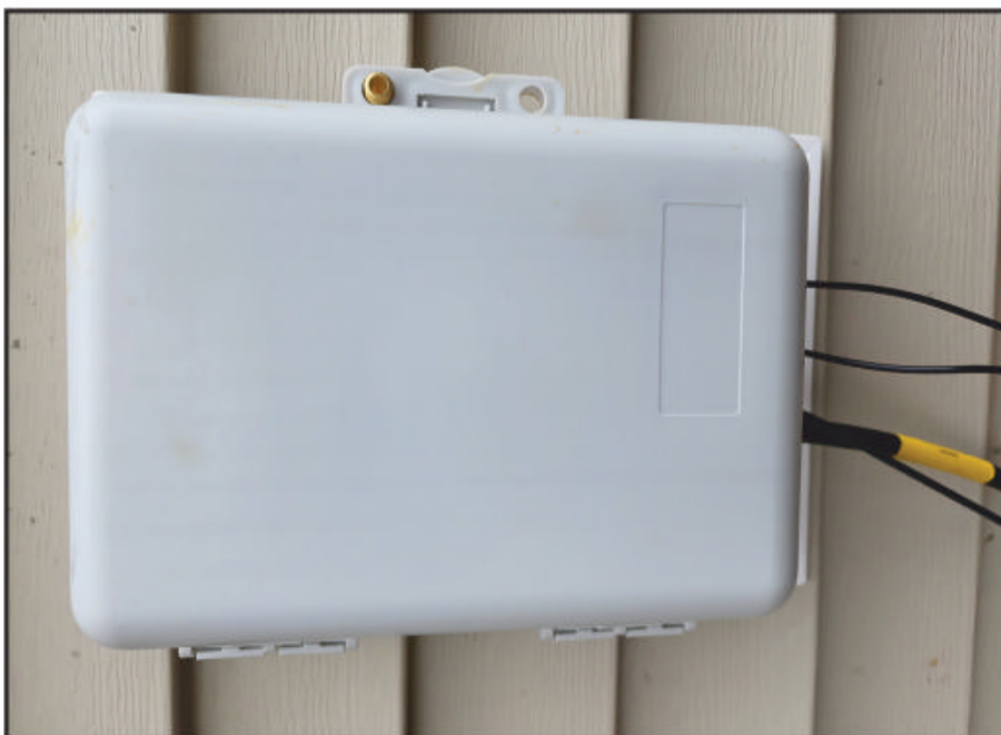
Photo G. NØBMK's finished exterior coax entrance. (Photo by NØBMK)
