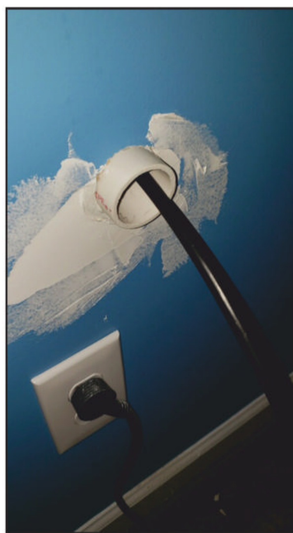
Photo D. Brian's interior wall with the 1.9-inch OD PVC pipe protruding into his shack. (Photo by NØBMK)
