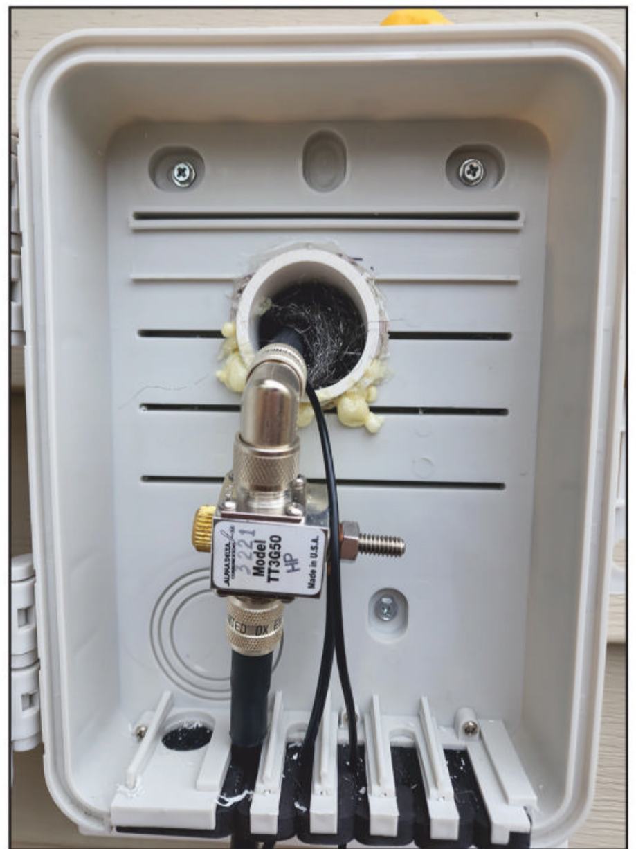
Photo H. Inside NØBMK's weatherproof enclosure. Note the Alpha Delta gas discharge lightning protector in line with the antenna coax and the grounding cables from the Alpha Delta and from the shack to an outside ground pipe. (Photo by NØBMK)
