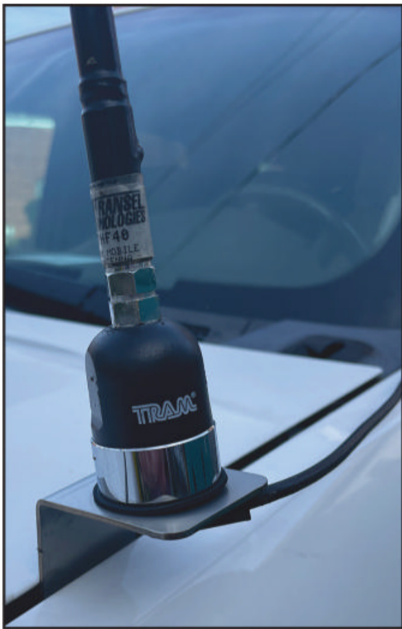
Photo B. A bracket mount on the hood of N4DTF's vehicle solved problems in his mobile installation caused by poor grounding.
