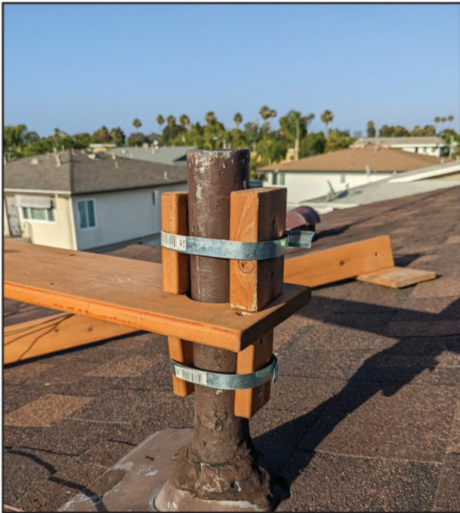
Photo B. The PVC vent pipe anchors the homebrew antenna base to the roof, avoiding the need to drill holes or drive nails through the roof.
