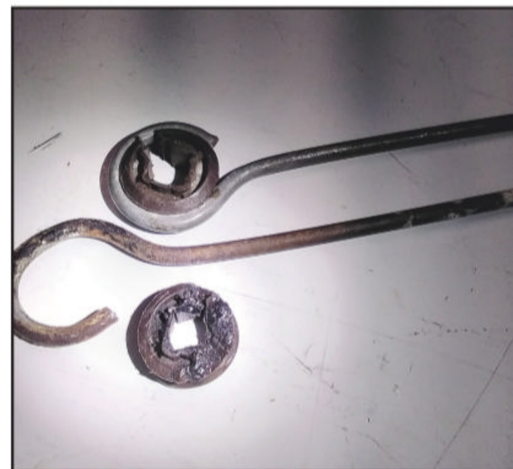
Here is the offending eyelet and insulator removed for inspection and replacement that is adjacent to one that appears to be intact but showing the signs of stress on the inner edge of the black plastic insulator. (Courtesy of W3TS)
