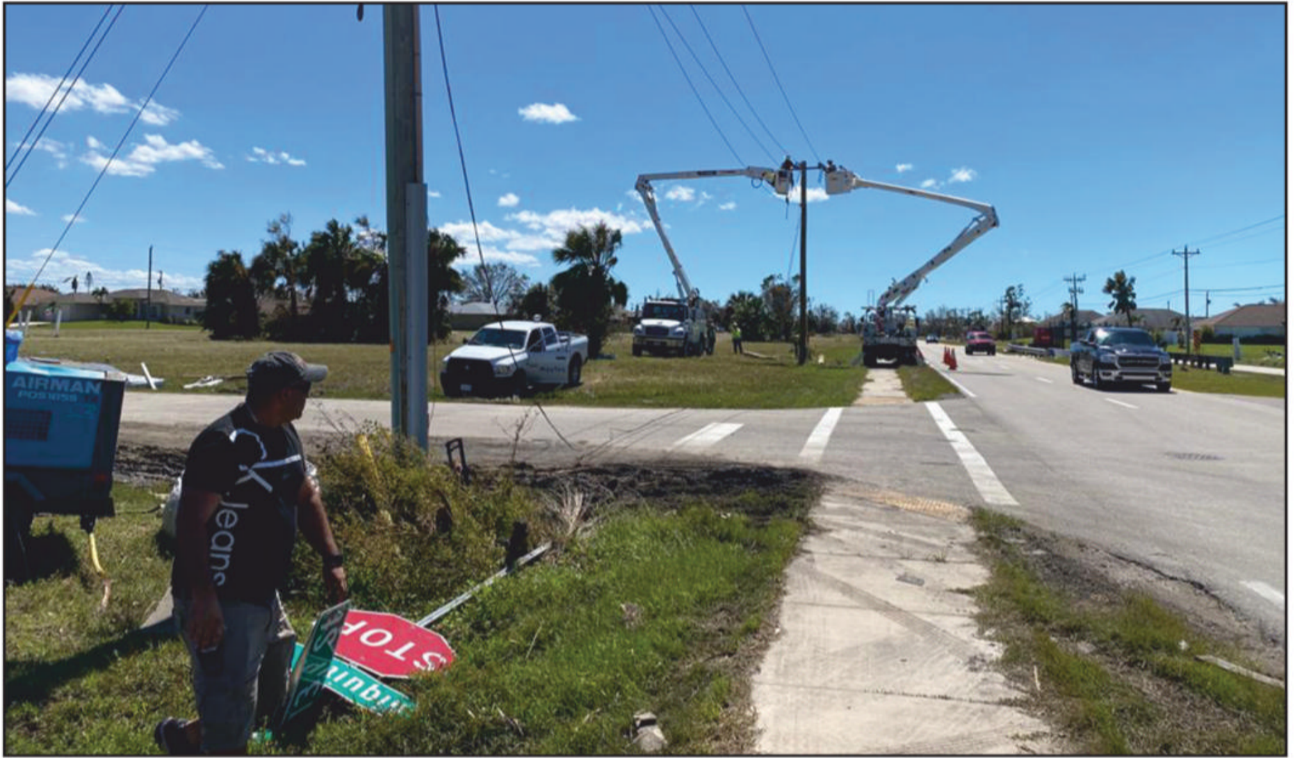
Utility crews work to restore power to storm-ravaged areas on Florida's west coast.
