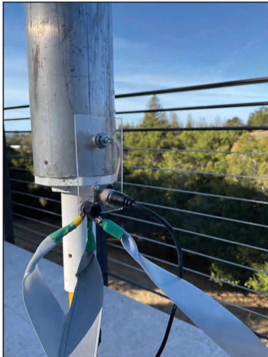
Photo M. Detail showing connection of feedline and computer-cable radials to the base of the antenna.
