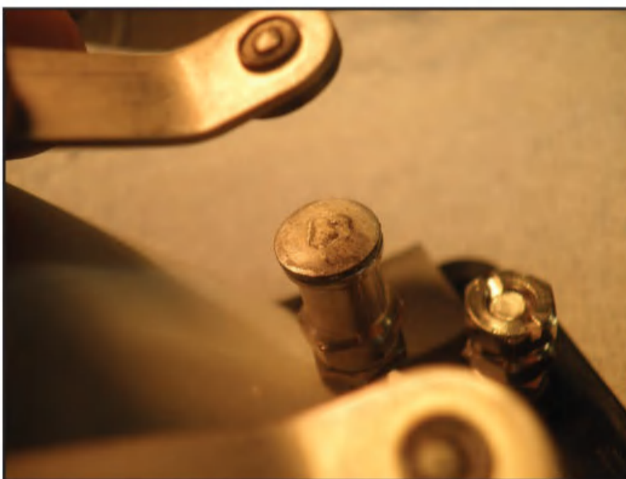
Photo A. White powdery residue from rosin flux can be hard to see on a switch contact — even with a magnifying glass — but can create a thin layer of insulation that prevents current from flowing.
