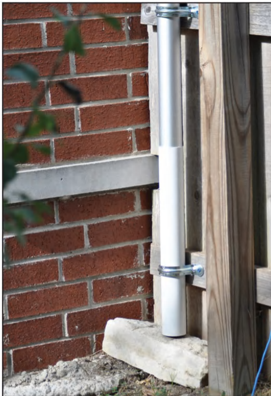
Photo B. The flagpole rests on a brick and is not buried.
