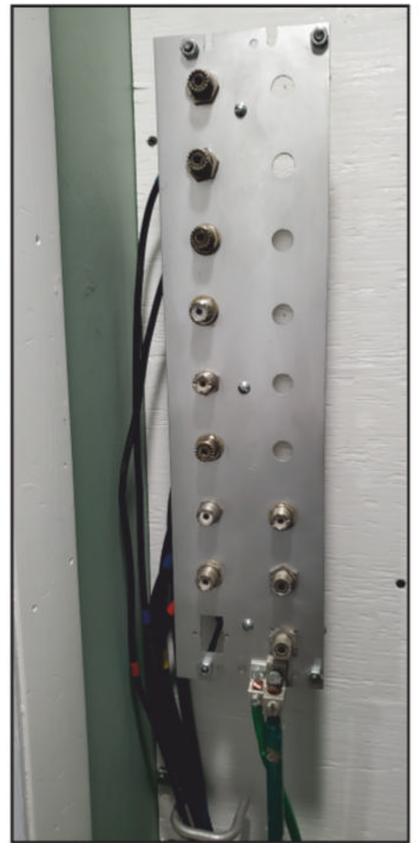
Photo D. Antenna patch panel makes swapping antennas and rigs easy.
