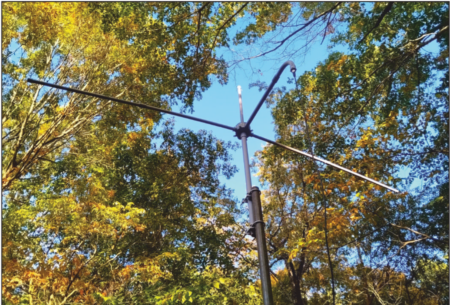
Photo F. The mast-mounted 6-meter / 2-meter / 70-centimeter tri-bander
