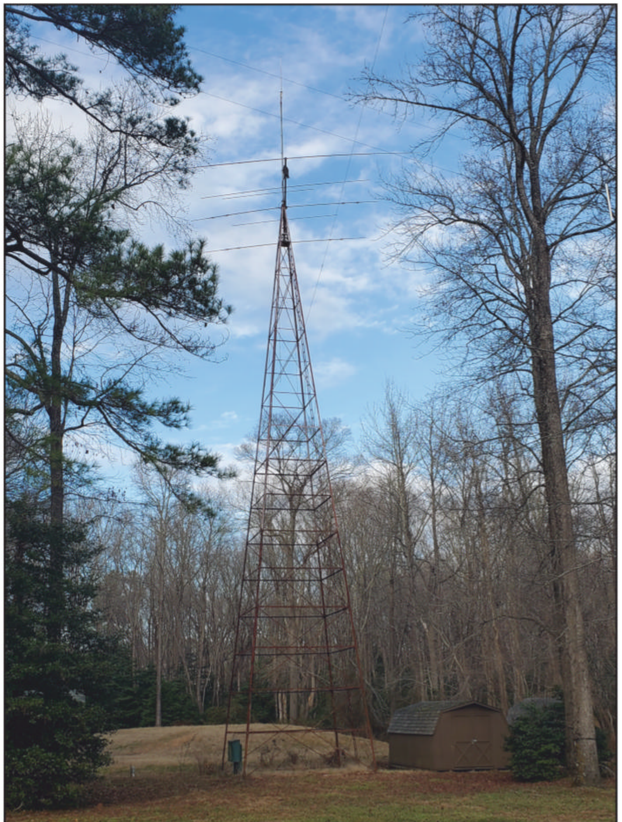
Photo A. Former windmill tower. All joints bolted like a large erector set. (All photos by K3PFW)
