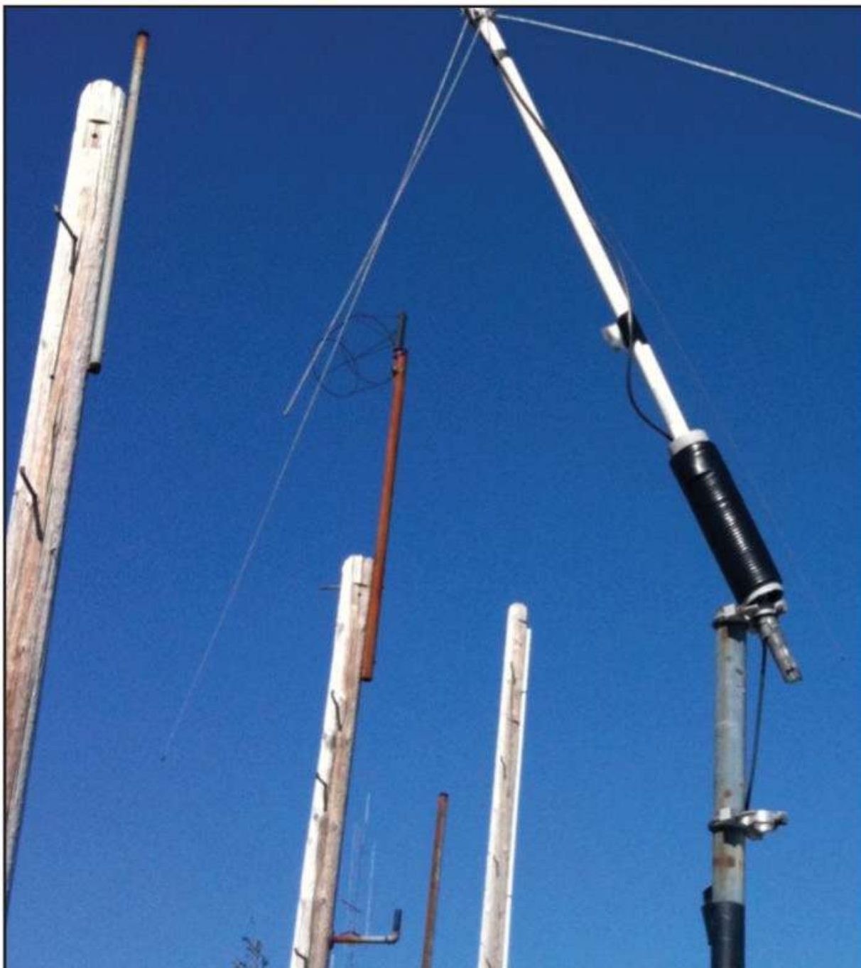
Photo C: W6WX beacon antenna damaged by wind. The beacon stations sometimes operate in very harsh weather conditions.
