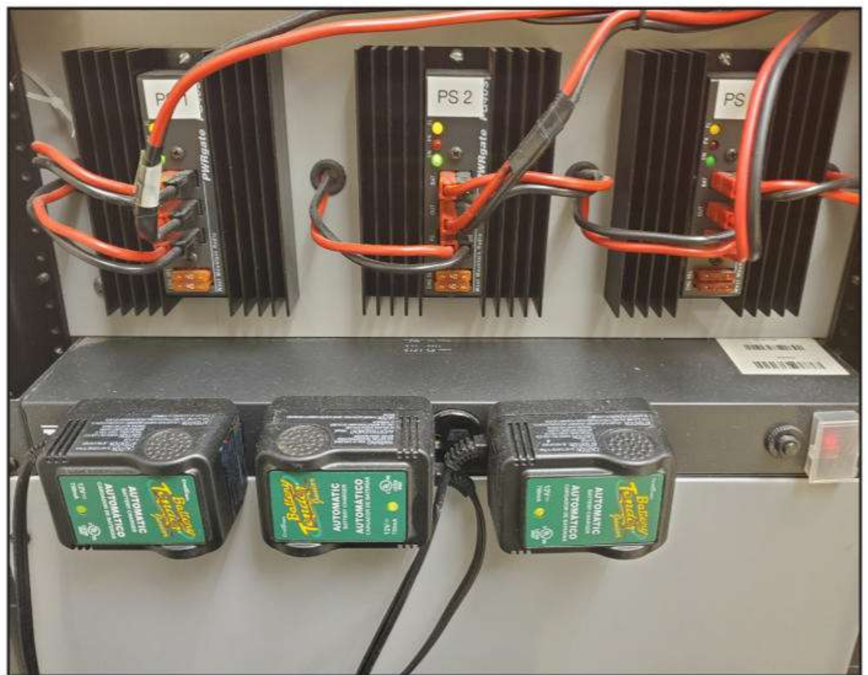
Photo B: The charge controllers allow the power supplies to operate the positions, with an instantaneous switch to battery in case of a power loss. They are out in plain sight so issues are spotted quickly.
