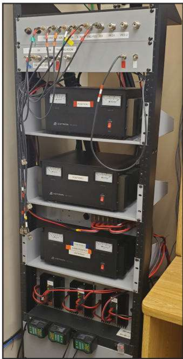
Photo A: “The Rack” in the amateur radio station at the Sussex County (DE) Emergency Operations Center (EOC). The three power supplies, associated charge controllers and batteries power the three operating positions. Redundancy allows for a quick switch and substitution if a failure occurs. Likewise, the antenna patch panel provides the flexibility to connect any radio to any antenna.
