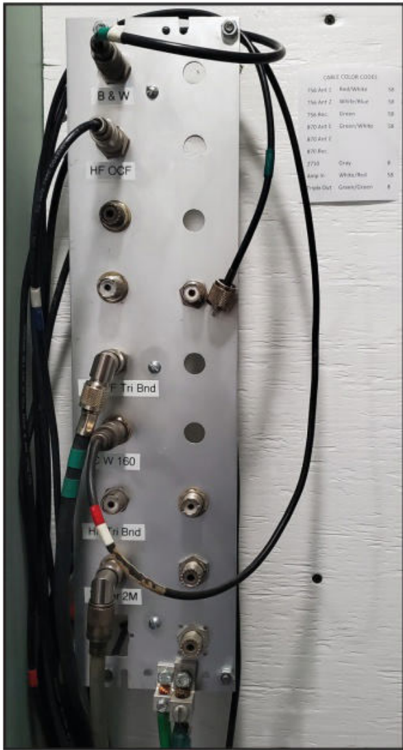
Photo B. Patch panel, tucked away in the closet, now populated with cables and labels.
