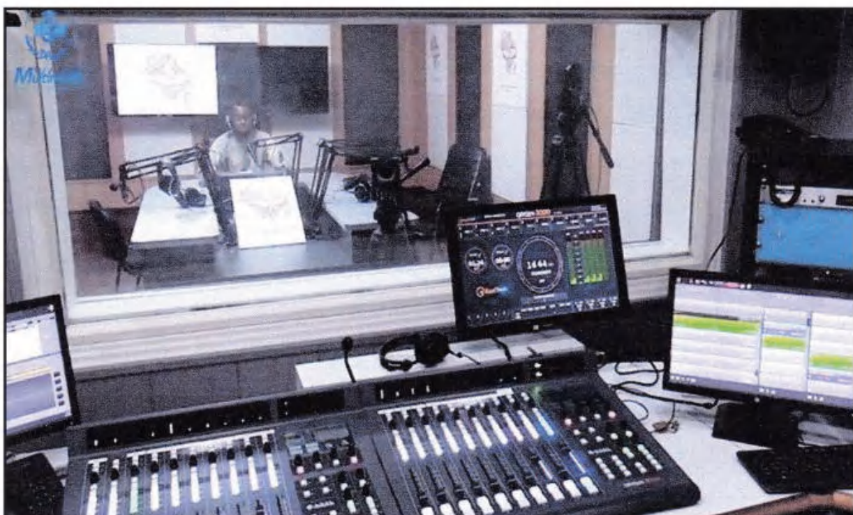
A control room at the new ifrikya FM in Algiers, Algeria.
