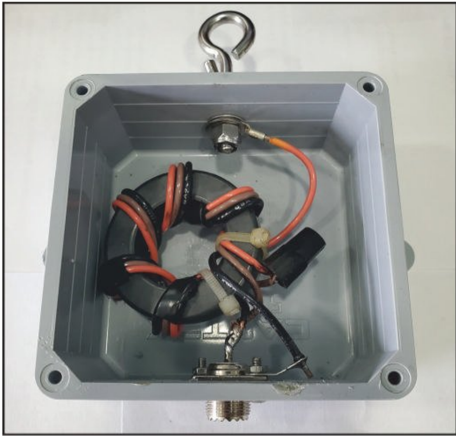
Photo C. The unun installed in its enclosure with connecting hardware
