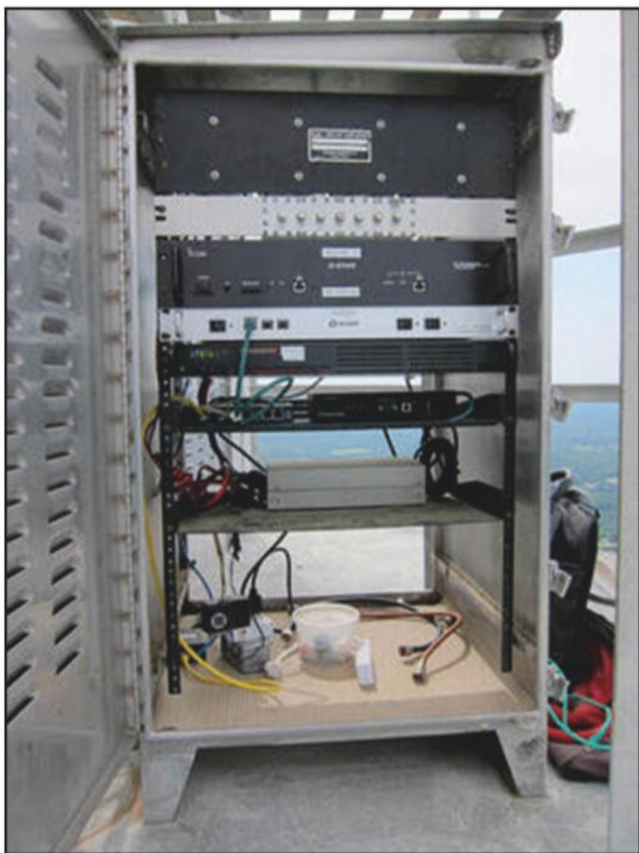
Photo C. An inside look at the KA4YMZ-A repeater
