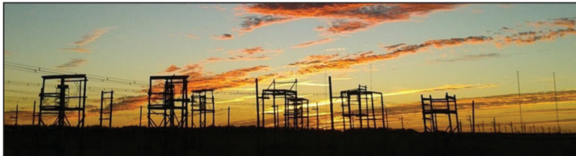
Here’s what’s left of the WRMI antennas after Hurricane Ian had its way.
