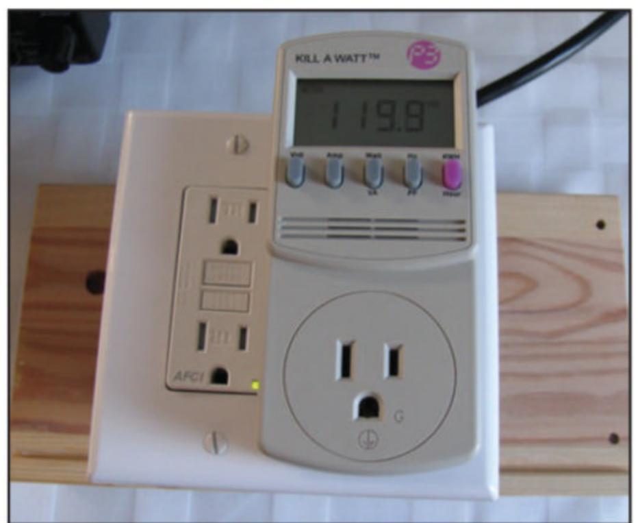
Photo G. I re-built the test setup and mounted the components on a scrap piece of wood. Now I can take this rig and test other stations and conditions to see how an AFCI would behave at different locations.
