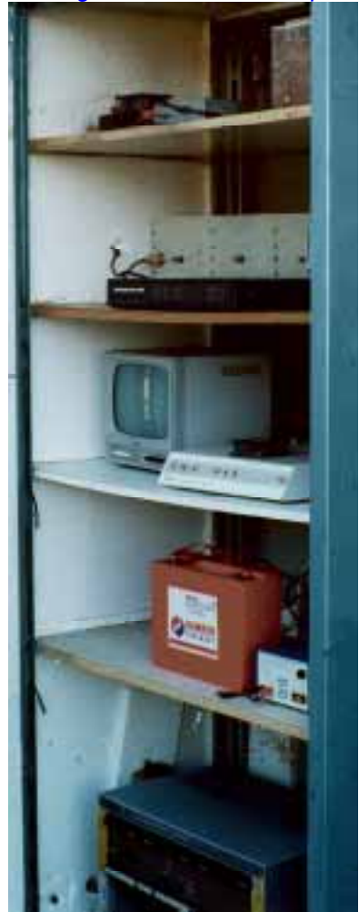
The Equipment Stack
