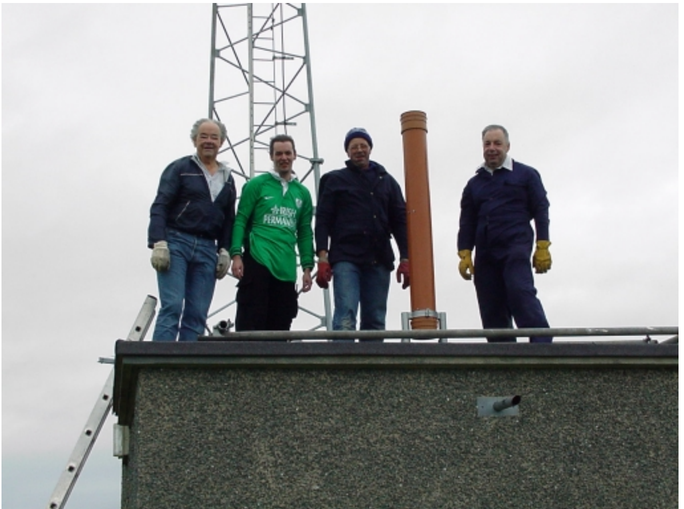
This photo shows the antenna installation crew for the forthcoming new ATV repeater (GB3GW located near Criccieth) which will cover the West coast of Wales & Cardigan Bay.
