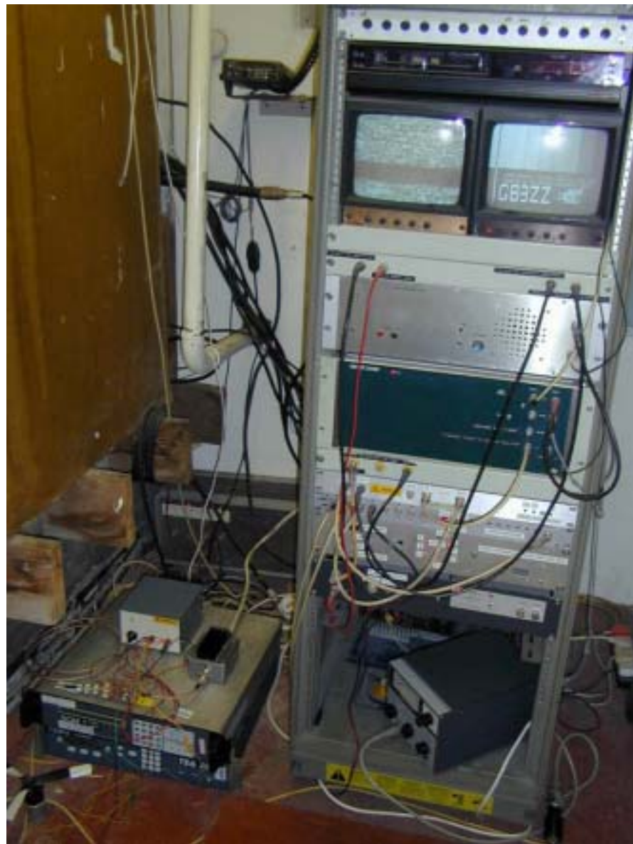
Transmit equipment in shack with GB3ZZ
